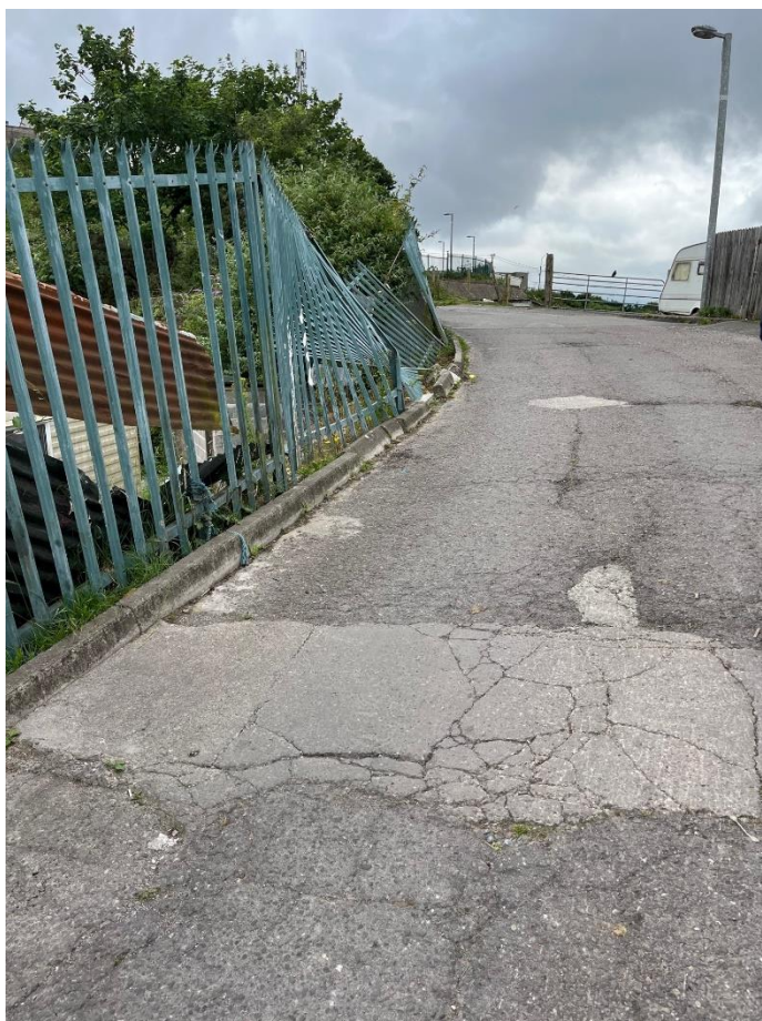
Figure 2-4 – Location of previous loss of control incident.
