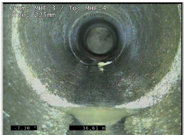
Joint displaced medium
