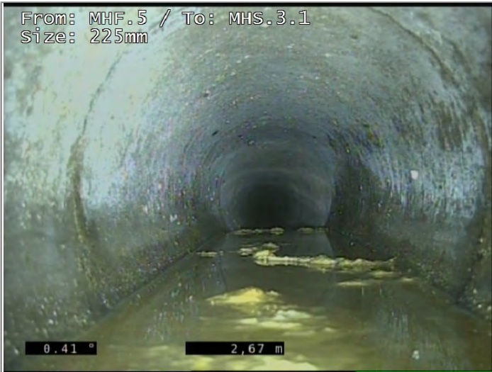
Debris 10% cross-sectional area loss
