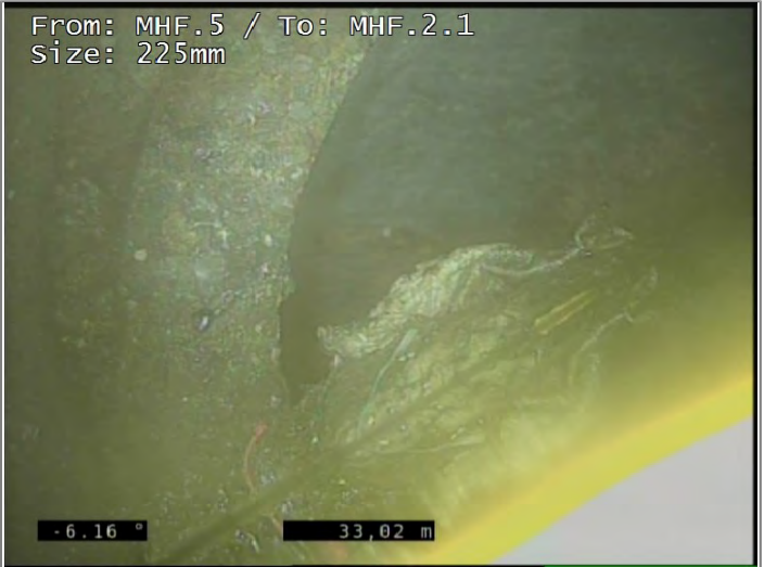
Line of sewer deviates left
