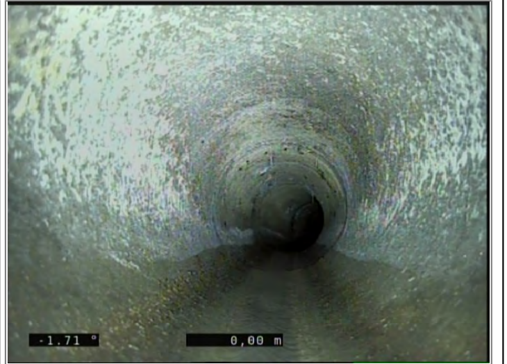
Start node type, manhole, reference MHS.1
