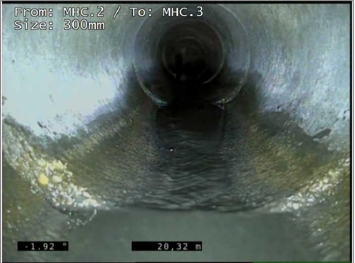
Joint displaced medium
