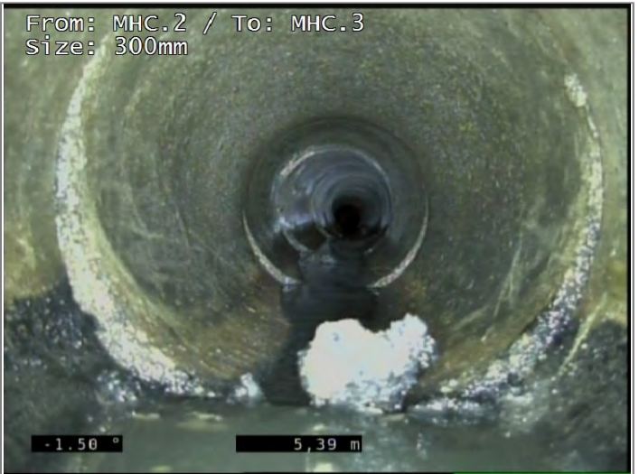
Line of sewer deviates right
