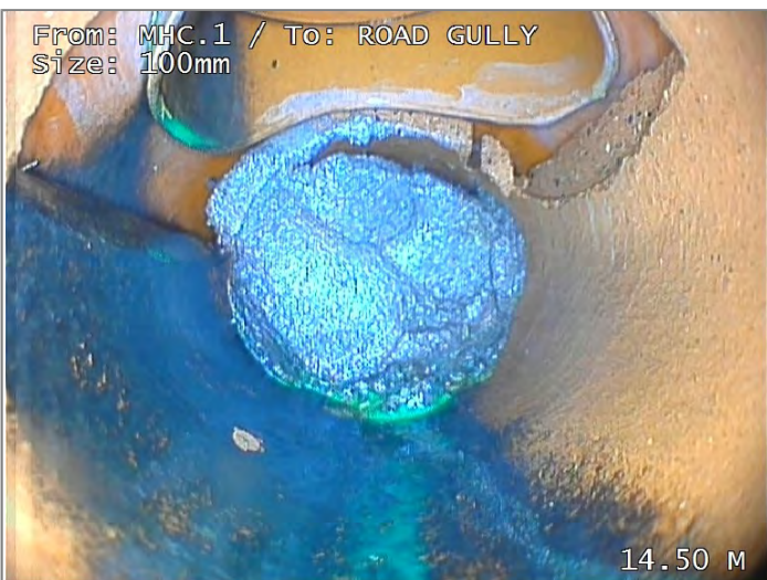
Connection at 12 o'clock, diameter 100mm - Remark: PVC.. GULLY IN CAR PARK.
