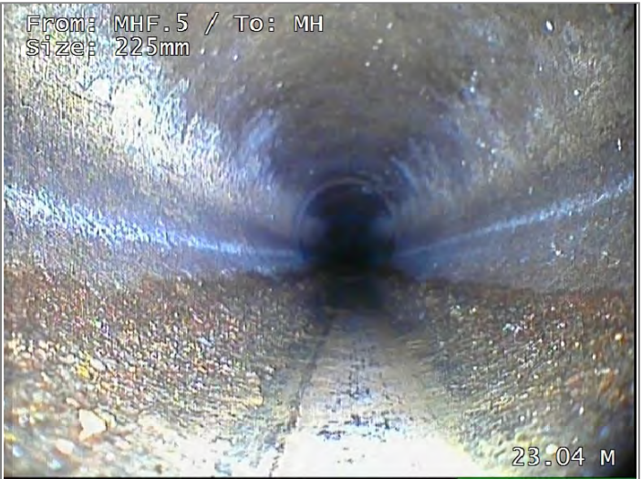
Survey abandoned - Remark: CAMERA WILL NOT TRAVEL.
