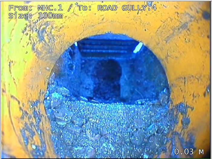
ROAD GULLY .4 IS LOCATED INSIDE THE ENTRENCE OF THE LIBRARY ON THE RIGHT HAND SIDE.
