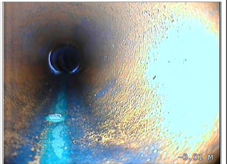
Start node type, manhole, reference MHC.1
