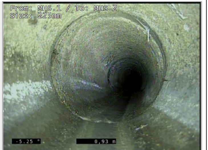
Line of sewer deviates right
