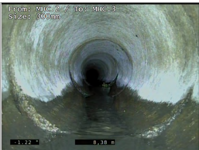
Joint displaced medium
