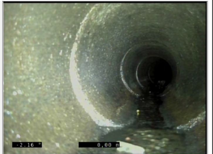
Start node type, manhole, reference MHC.2
