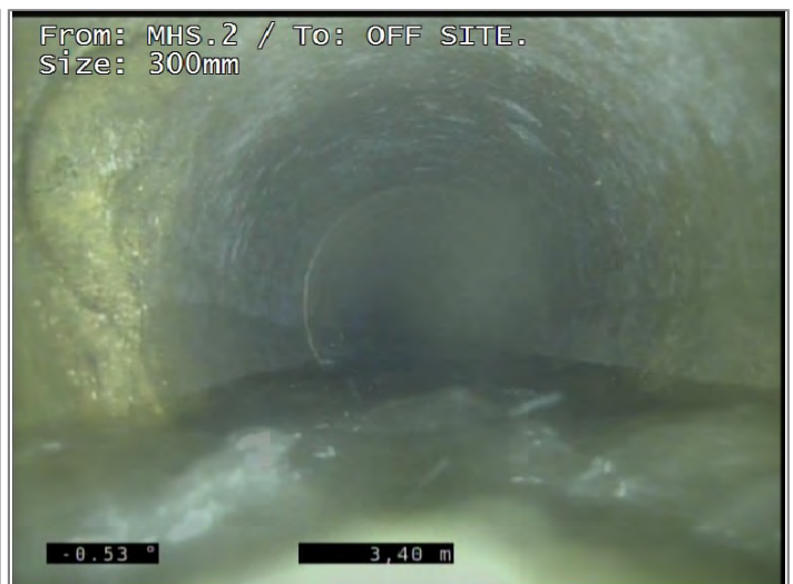
From: MHS.2 / To: OFF SITE. Size: 300mm Connection at 9 o'clock, diameter 100mm - Remark: EW
