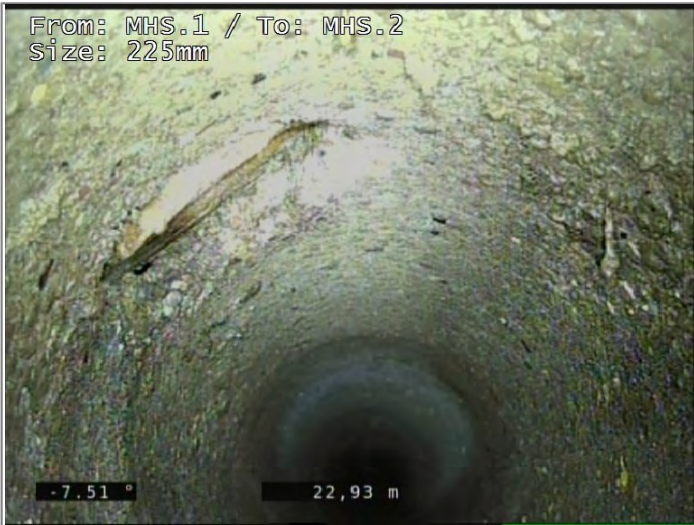
Connection at 10 o'clock, diameter 100mm - Remark: EW
