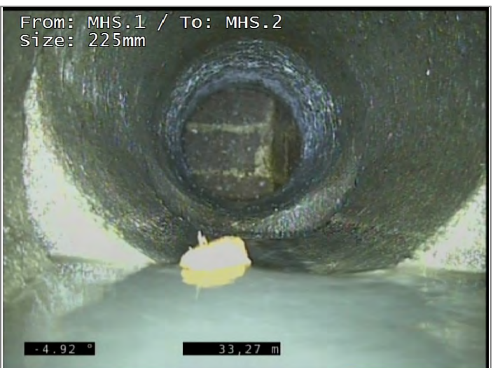
Joint displaced medium
