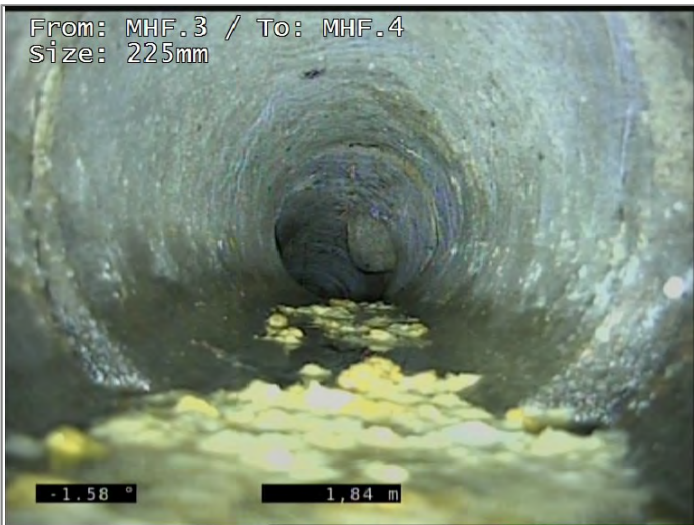
Joint displaced medium
