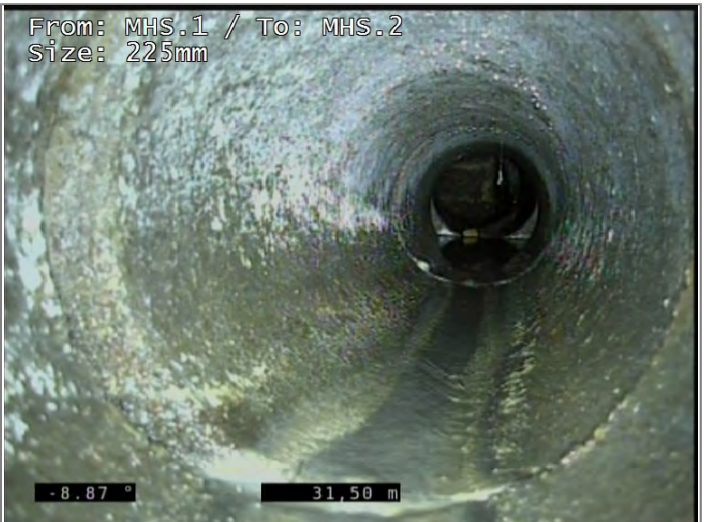
Joint displaced medium
