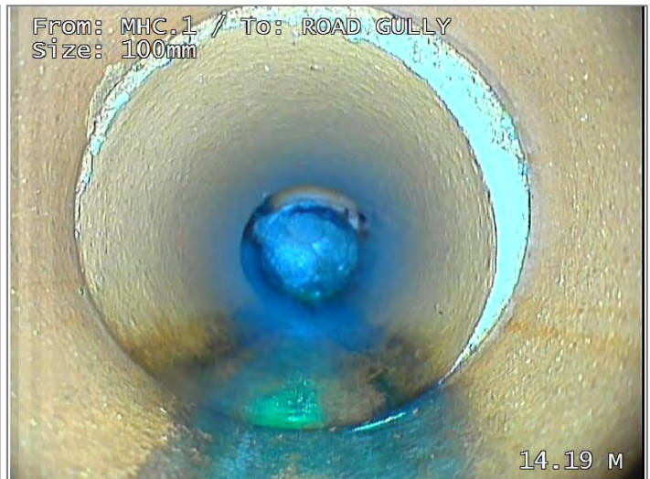
Joint displaced medium
