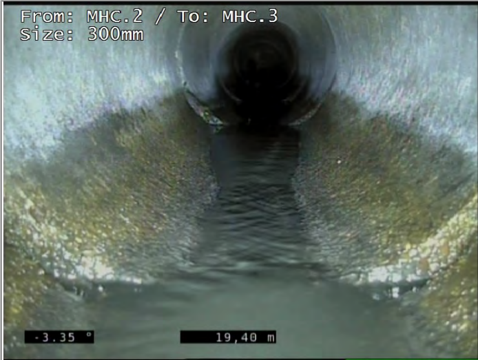
Joint displaced medium
