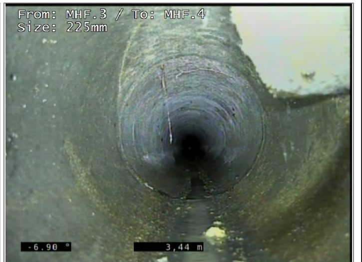
Connection at 2 o'clock, diameter 100mm, intrusion 25mm
