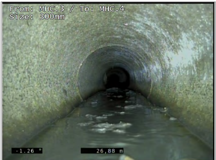
Debris 15% cross-sectional area loss
