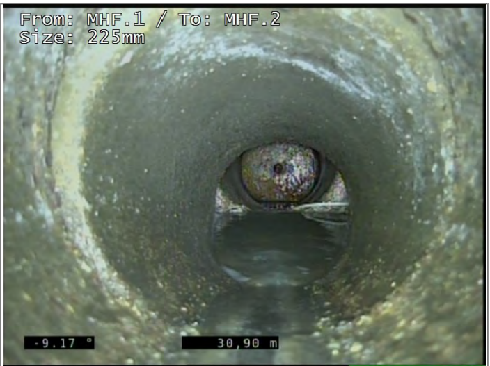
Joint displaced medium
