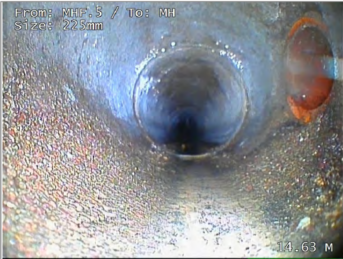
Connection at 3 o'clock, diameter 100mm - Remark: EW
