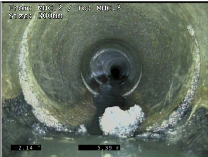
Joint displaced medium
