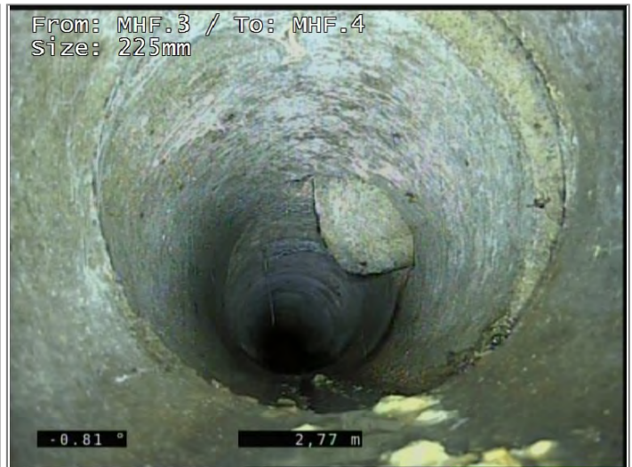
Line of sewer deviates down
