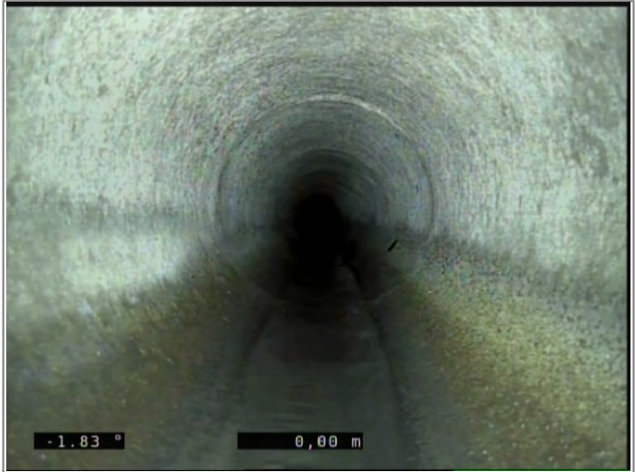
Start node type, manhole, reference MHC.3
