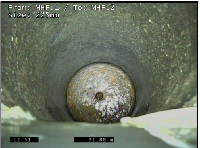
Line of sewer deviates down
