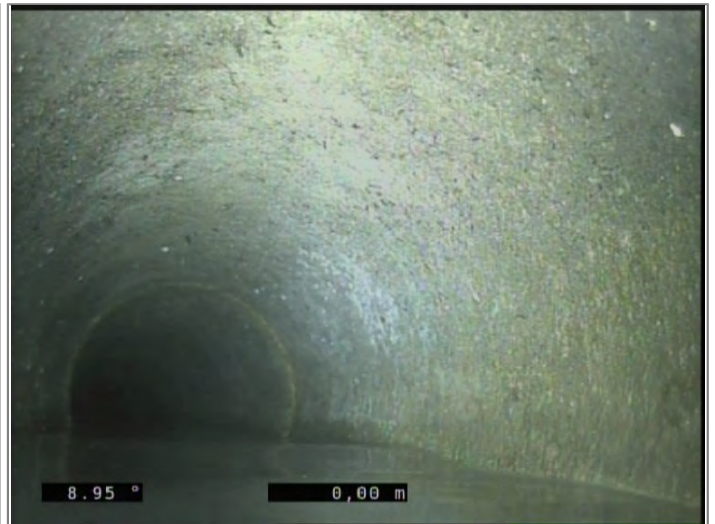
Start node type, manhole, reference MHS.2
