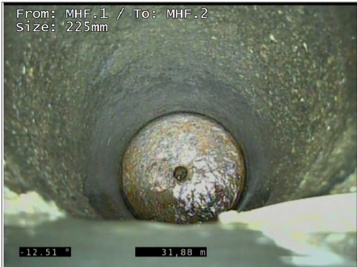
Joint displaced medium
