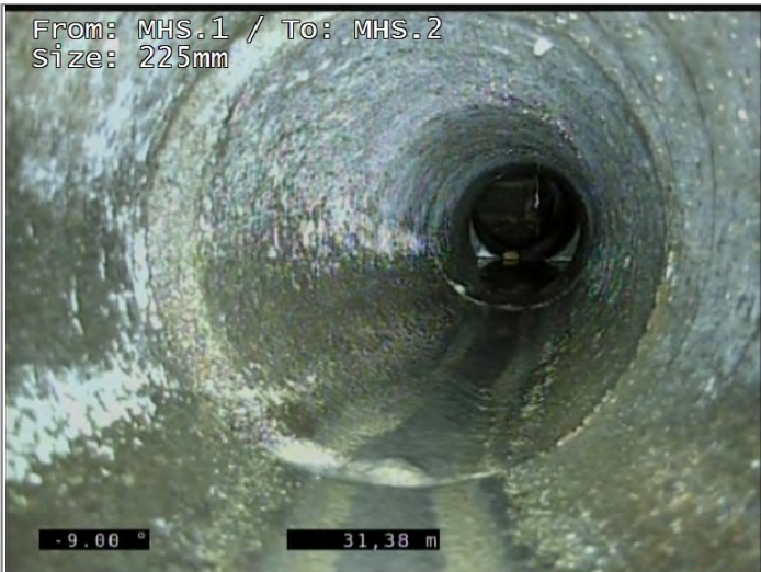
Line of sewer deviates right
