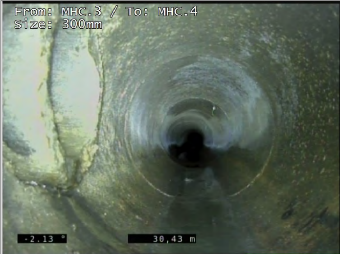
Survey abandoned - Remark: CAMERA WILL NOT PASS CONNECTION INTRUSION.
