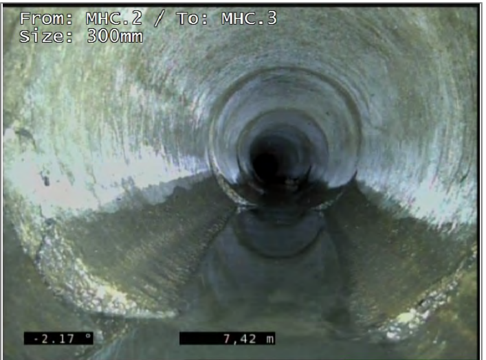
Joint displaced medium
