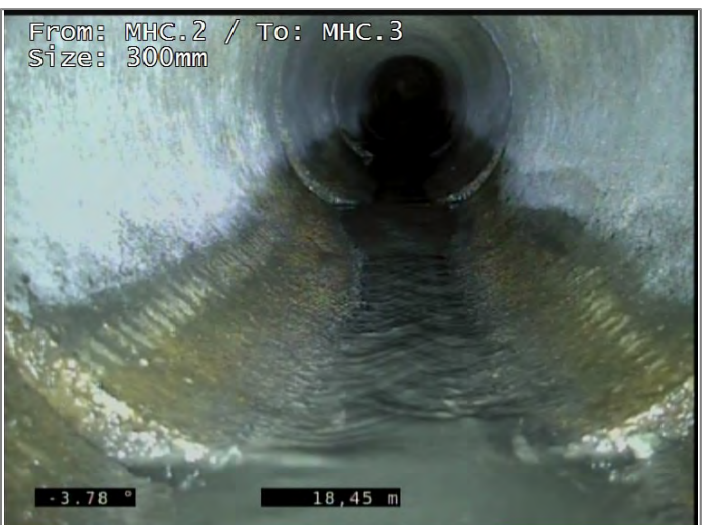
Joint displaced medium
