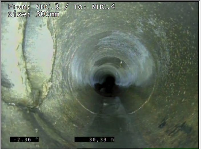
Connection at 9 o'clock, diameter 150mm, intrusion 25mm
