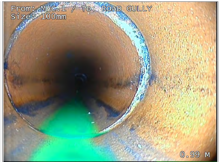
Joint displaced medium
