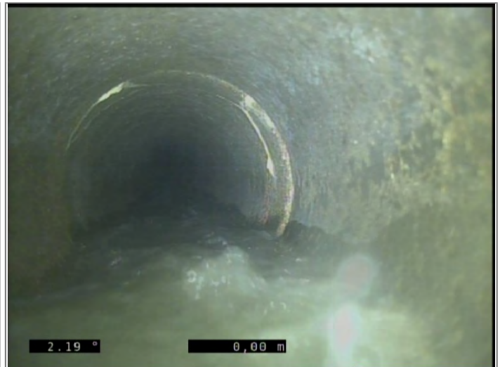
Start node type, manhole, reference MHS.2
