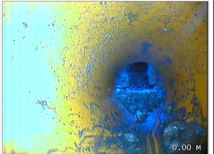
Start node type, manhole, reference MHC.1
