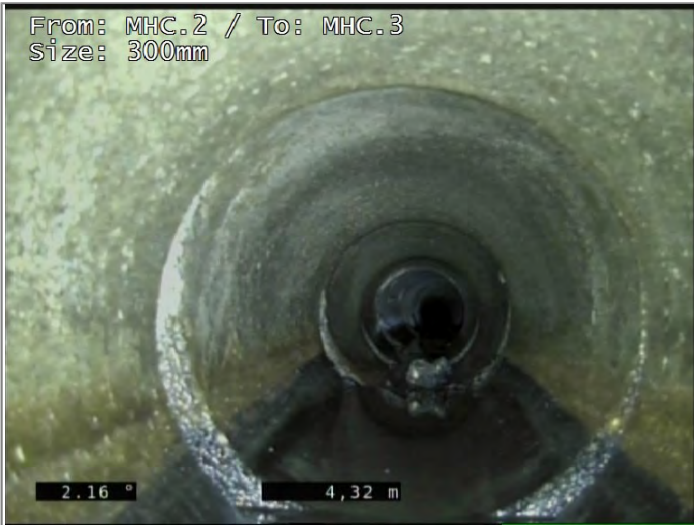
Joint displaced medium
