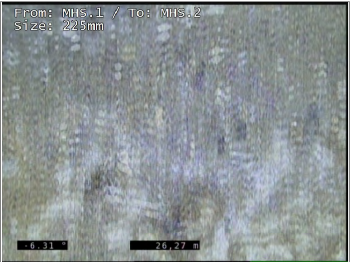
Connection at 12 o'clock, diameter 100mm - Remark: EW
