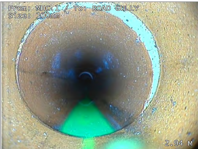
Joint displaced medium
