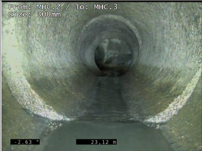
Joint displaced medium
