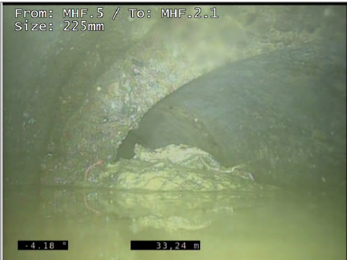
Debris 40% cross-sectional area loss - Remark: LINE WOULD NEED TO BE HIGH JETTED AND DEBRIS REMOVED FROM DRAIN TO CARRY OUT THE REST OF THE SURVEY.
