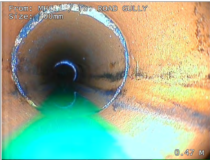
Joint displaced medium
