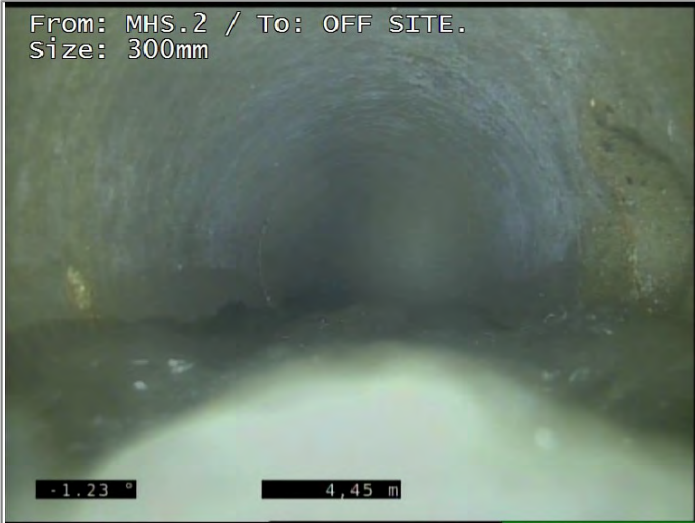
Connection at 3 o'clock, diameter 100mm - Remark: EW
