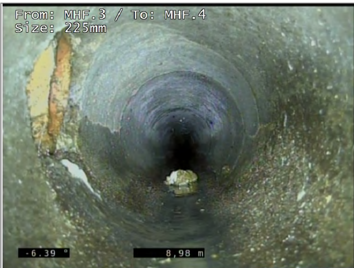
Connection at 9 o'clock, diameter 100mm - Remark: EW
