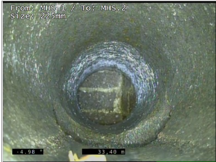
Line of sewer deviates down - Remark: DROR SHAFT INTO MHS.2
