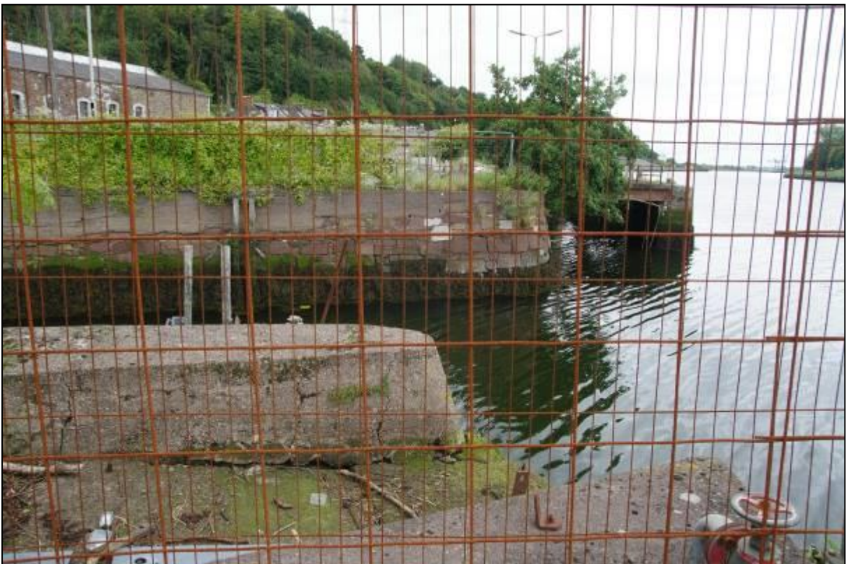
Plate 18: View of west facing side of south end of slipway (CHC 6) from west with section of wharf extending to east visible on right side
