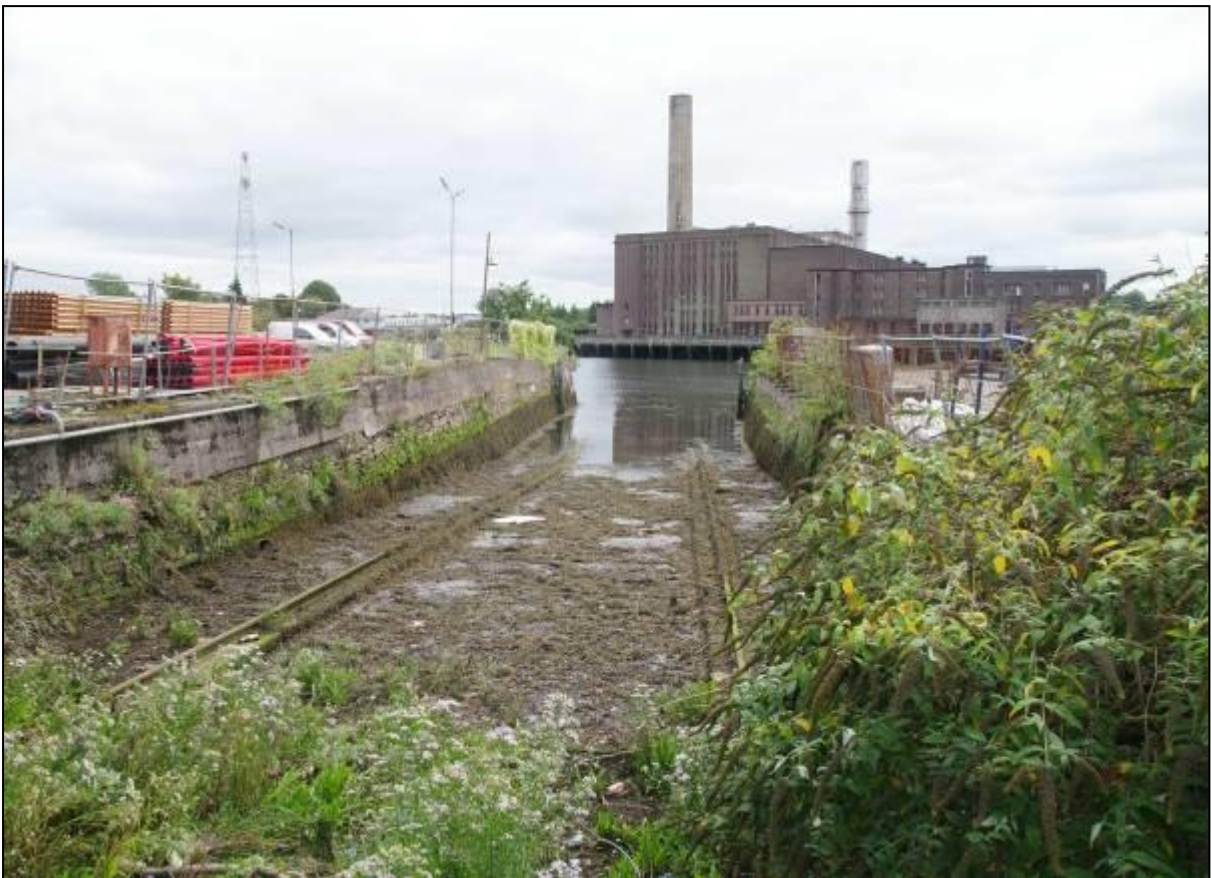
Plate 16: View of remaining slipway (CHC 6) within yard from northwest with concrete repairs to upper section of sidewalls and basal slideways visible
