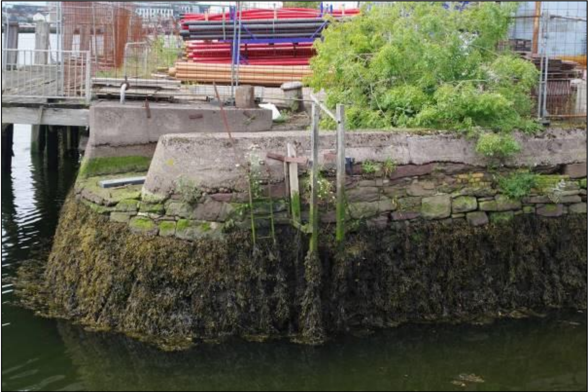
Plate 17: View of east facing side of south end of slipway (CHC 6) from east showing visible traces of random rubble construction and concrete repairs to upper section
