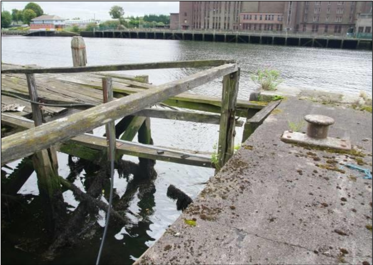
Plate 19: View collapsing section of wharf located to east of slipway (CHC 6) which is outside scheme boundary
