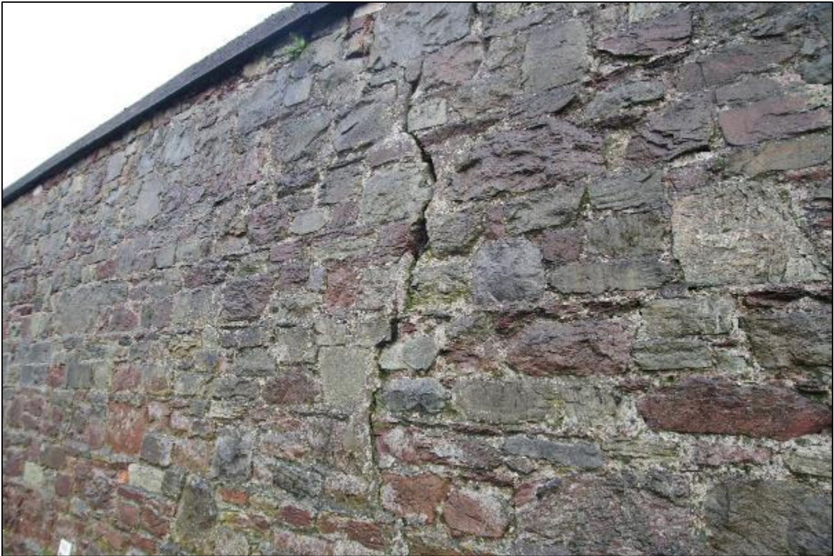
Plate 11: Detailed view of random rubble boundary wall showing crack in central area
