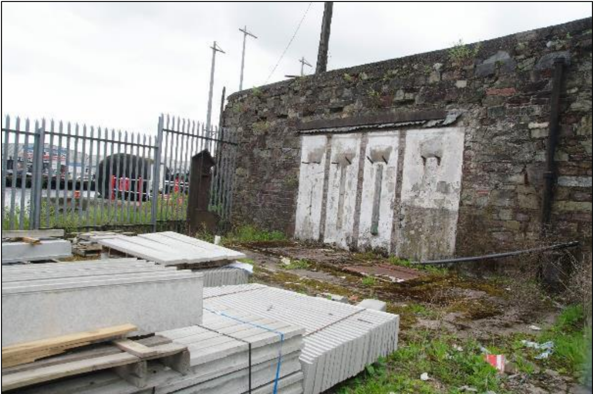
Plate 13: View of extant section of McMahon Builder Provision boundary wall on Water Street from east showing traces of removed concrete attached structure
