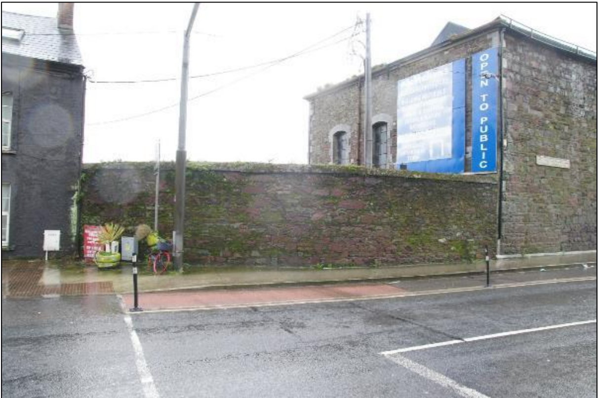
Plate 24: View from north of section of northern boundary wall of McMahon yard to be removed with workshop (CHC 7) visible on right side of frame
