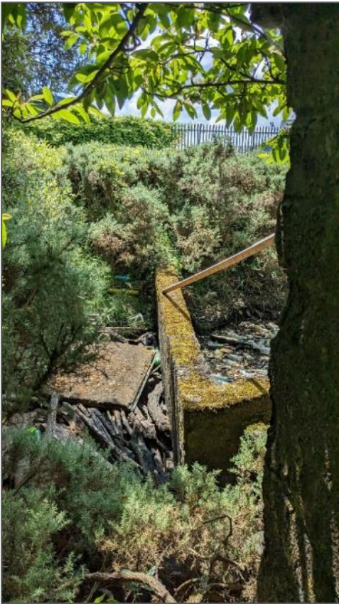
Plate 4-25 – Dry weir identified with large quantity of debris including vegetation, litter, household items (Coordinates: 51.905920, -8.400197)
