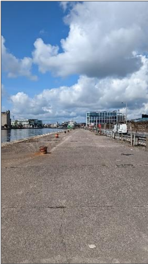
Plate 4-1 - Existing Quay where scarifying will be required prior to laying of blacktop.
