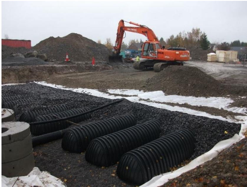
Figure 4-2: Typical attenuation/soakaway structure
