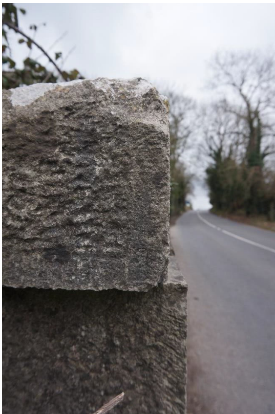
Parapet stone has shifted out of alignment on Northern end
