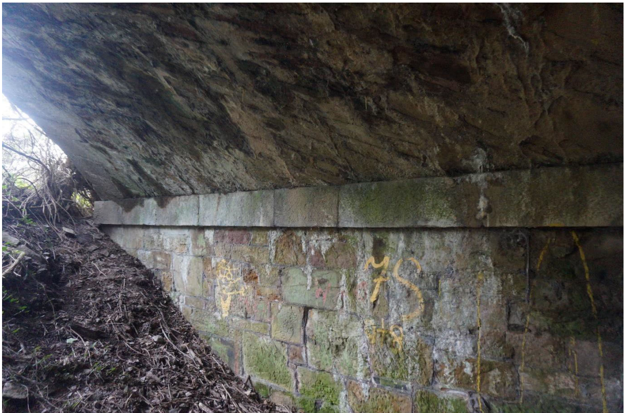
Detail of arch barrel rising from ashlar pier. Arch vault stonework is laid in a diagonal pattern and appears in good condition with mortar joinwork generally intact.
