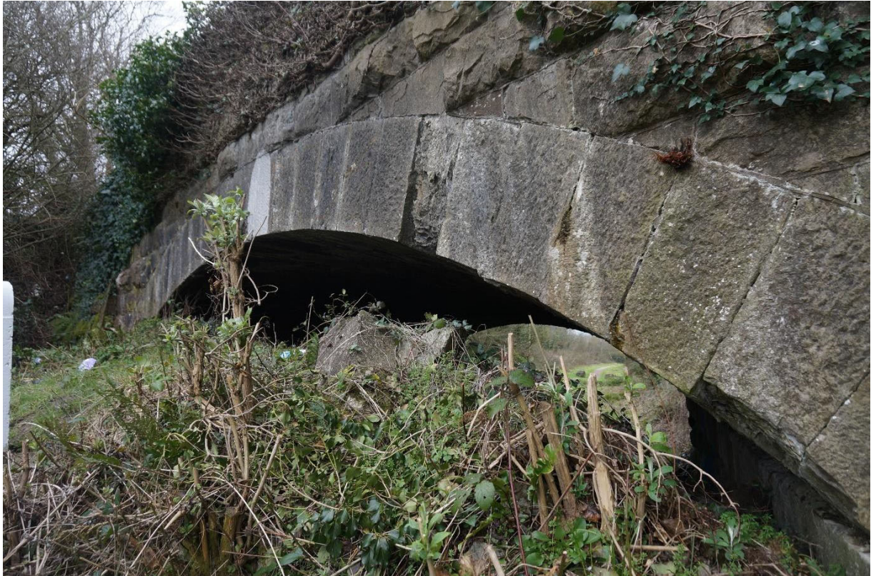
Surface damage to arch stones where earth mound built up to underside
