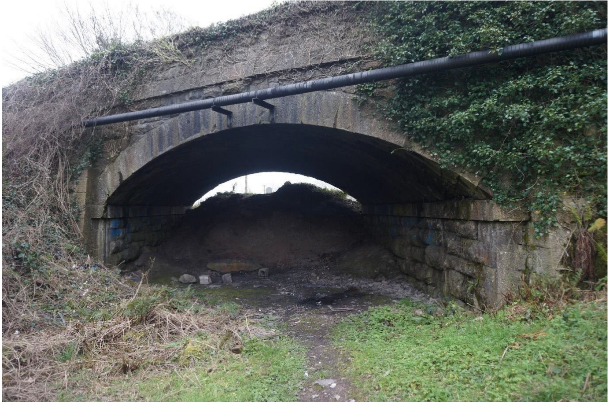
West elevation. Note invasive vegetation and ivy overburden
