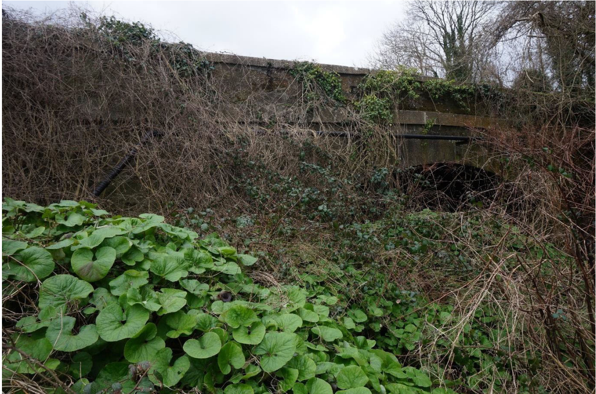
West elevation: Considerable vegetation overburden
