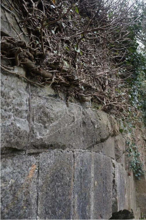
Severe invasive ivy growth beneath east parapet above arch
