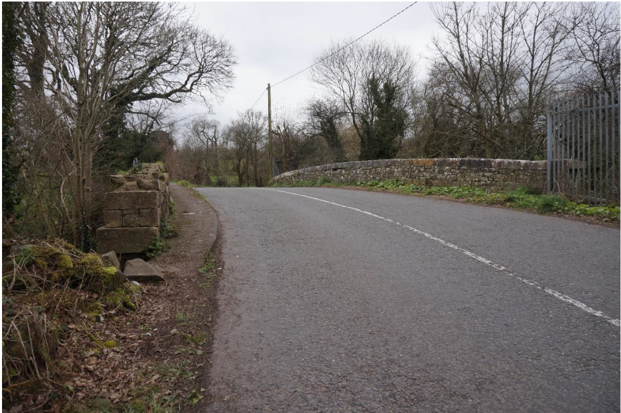
Approach road. Note intact parapet coping to East side and severe loss of stone to West
