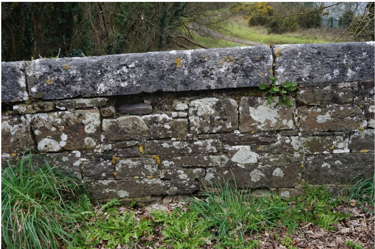
Local loss of stone beneath copings
