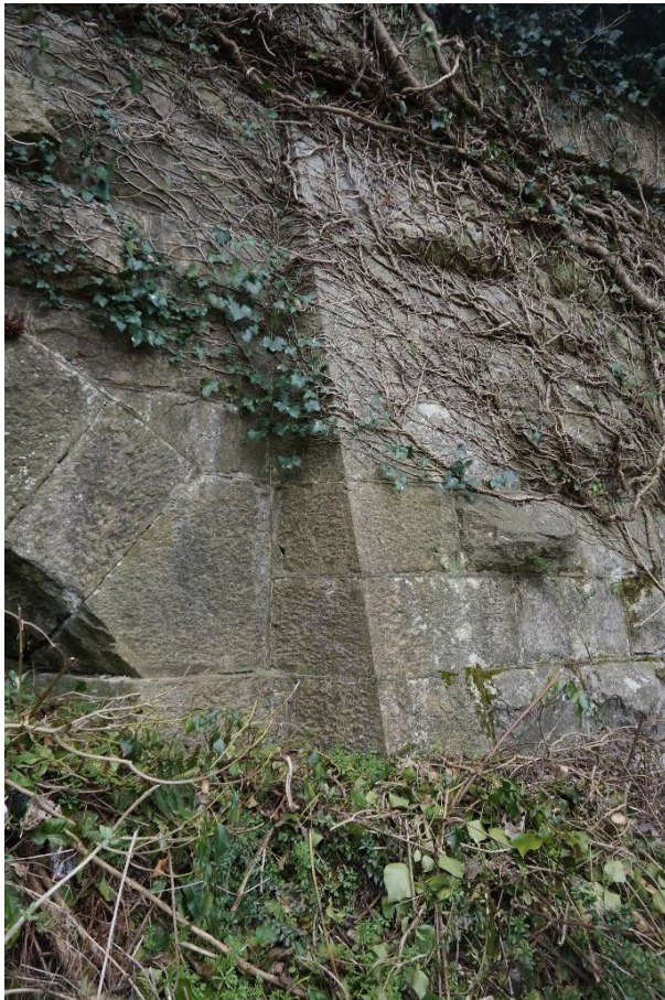
Considerable ivy tendrils present on abutment and wing walls
