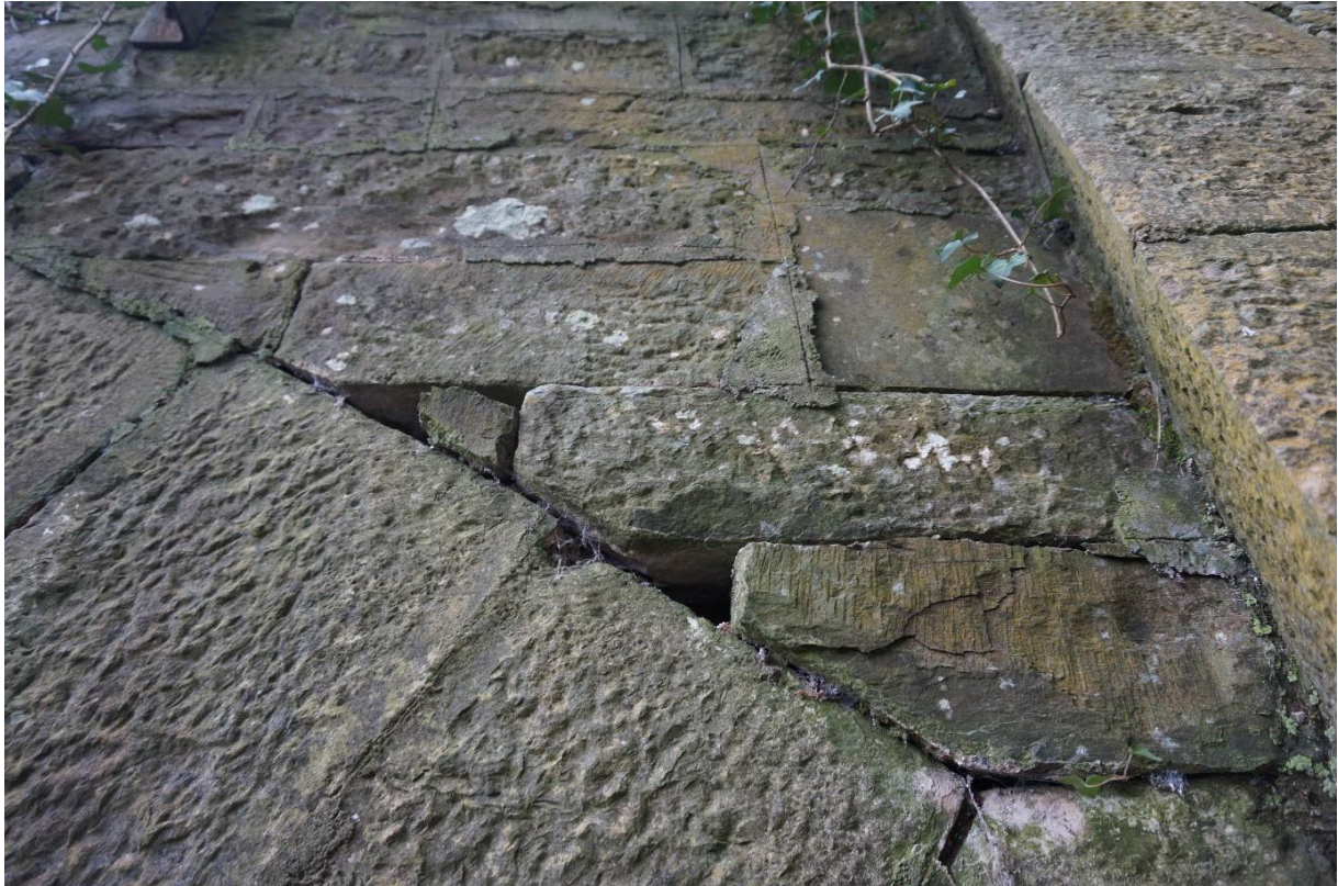
Loss of smaller stone pinnings above arch voussoirs
