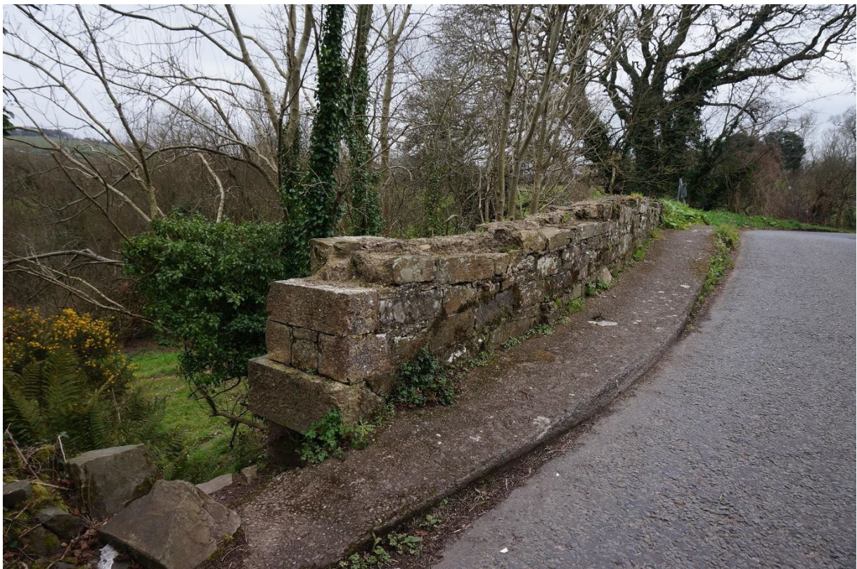
Loss of ashlar coping along flank of parapet and ashlar pier
