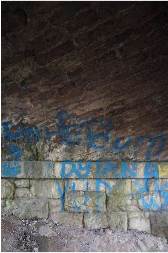
Arch barrel stone is laid in a diagonal pattern and is largely intact with some leeching of salts from mortar joints. Note heavy graffiti and loss of mortar from pier joints
