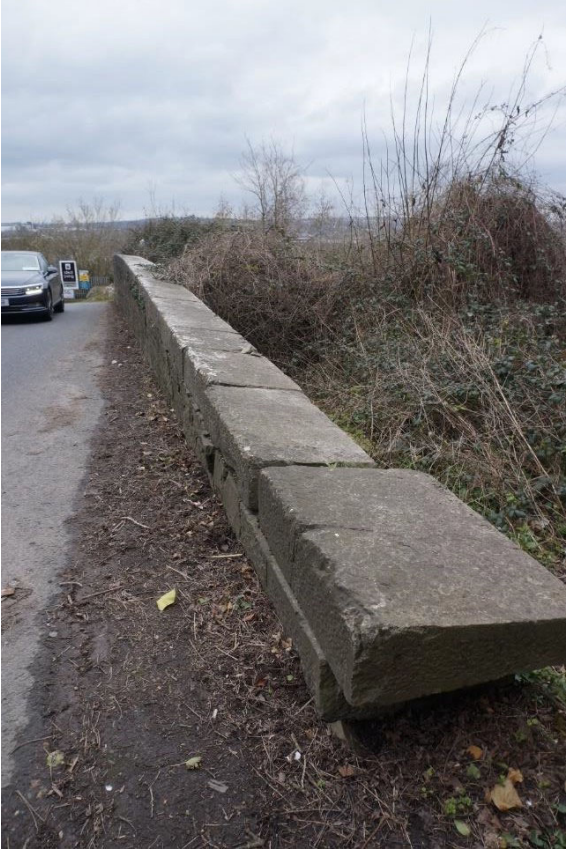
Loose and unconsolidated parapet capping stones
