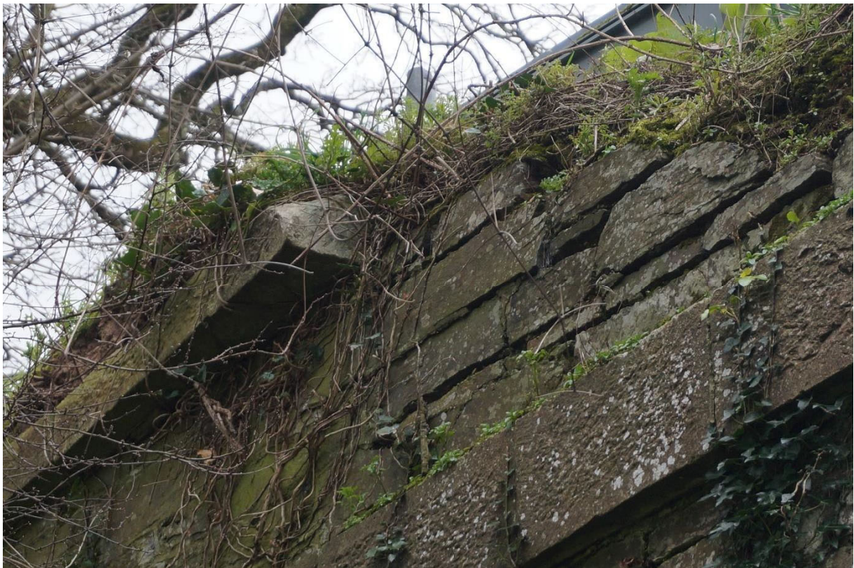
Missing and dislodged parapet copings. Note buckling of spandrel wall stones and loss of pointing
