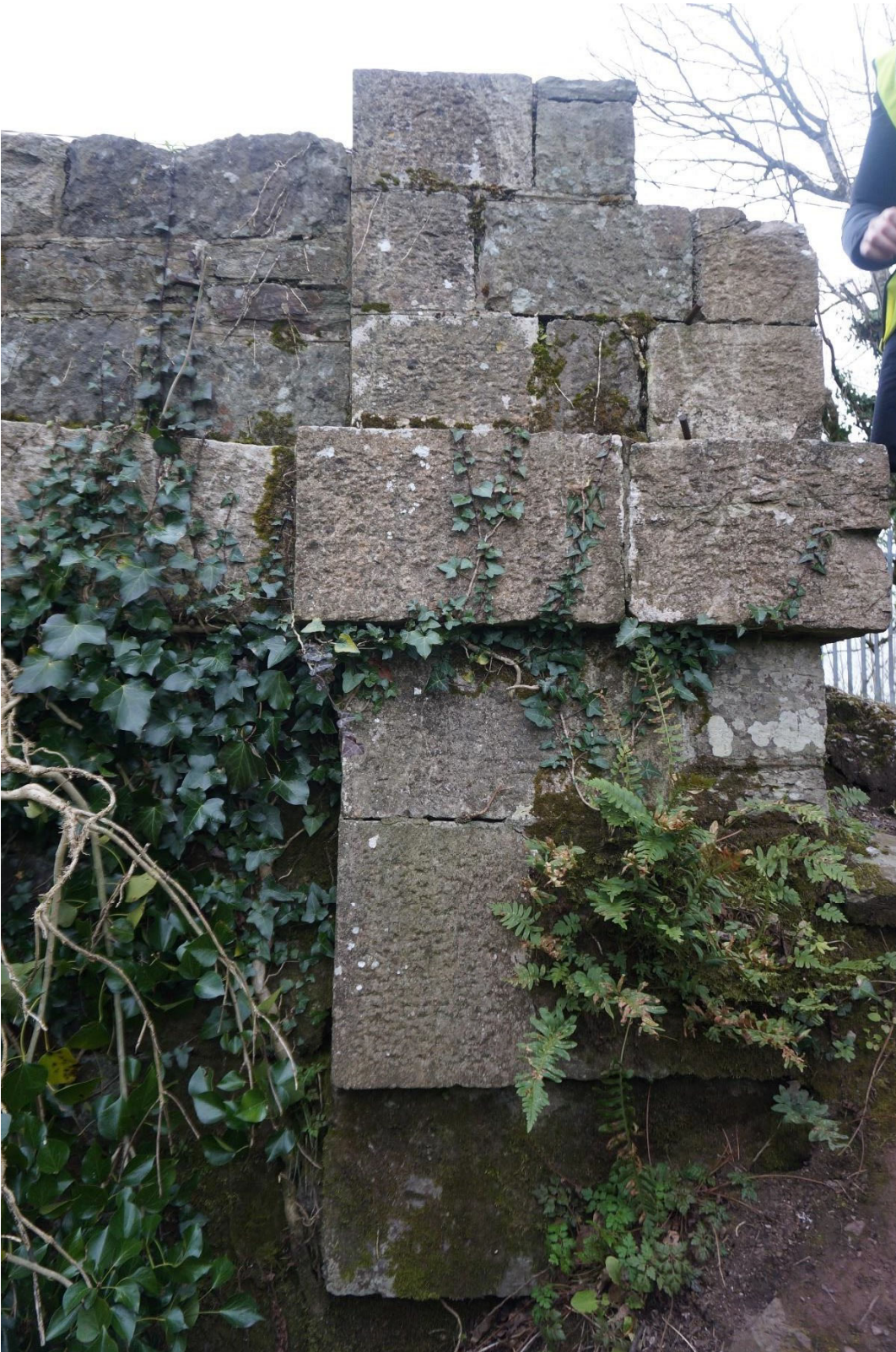
Abutment pier with severe loss of ashlar stone and parapet coping
