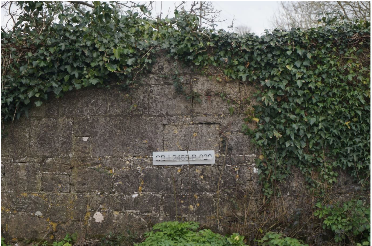
General roadside parapet elevation with loss of pointing to many stonework joints
