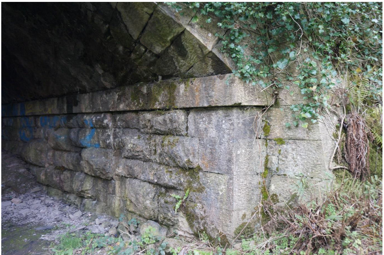
Heavy carbon soiling of stonework
