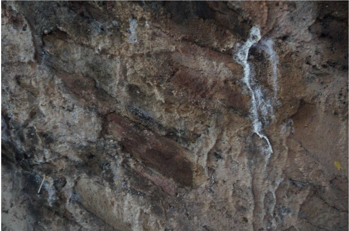
Some leaching of salts through arch barrel possibly from unsealed road surface
