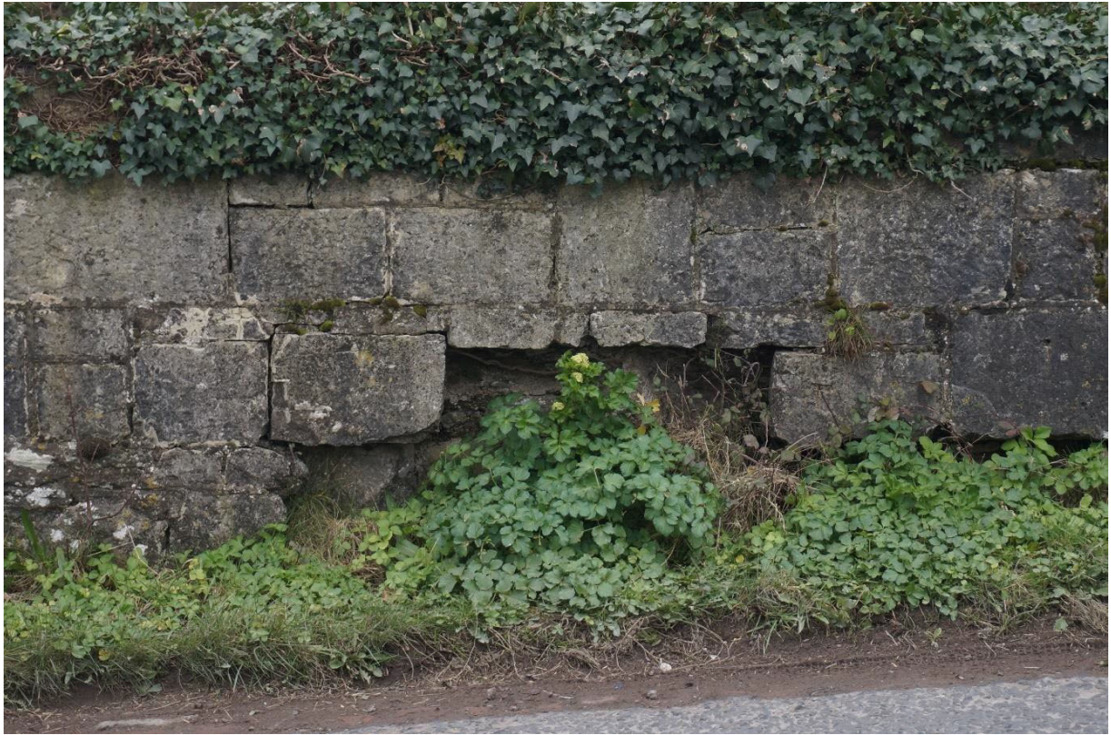
Loss of block limestone to East parapet on roadside
