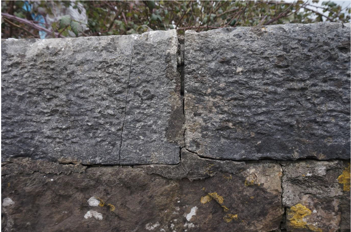
Loose and friable pointing mortars. Later replacement mortars are cement based
