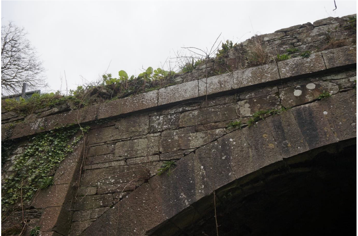
Missing, loose unconsolidated parapet stone with open jointwork
