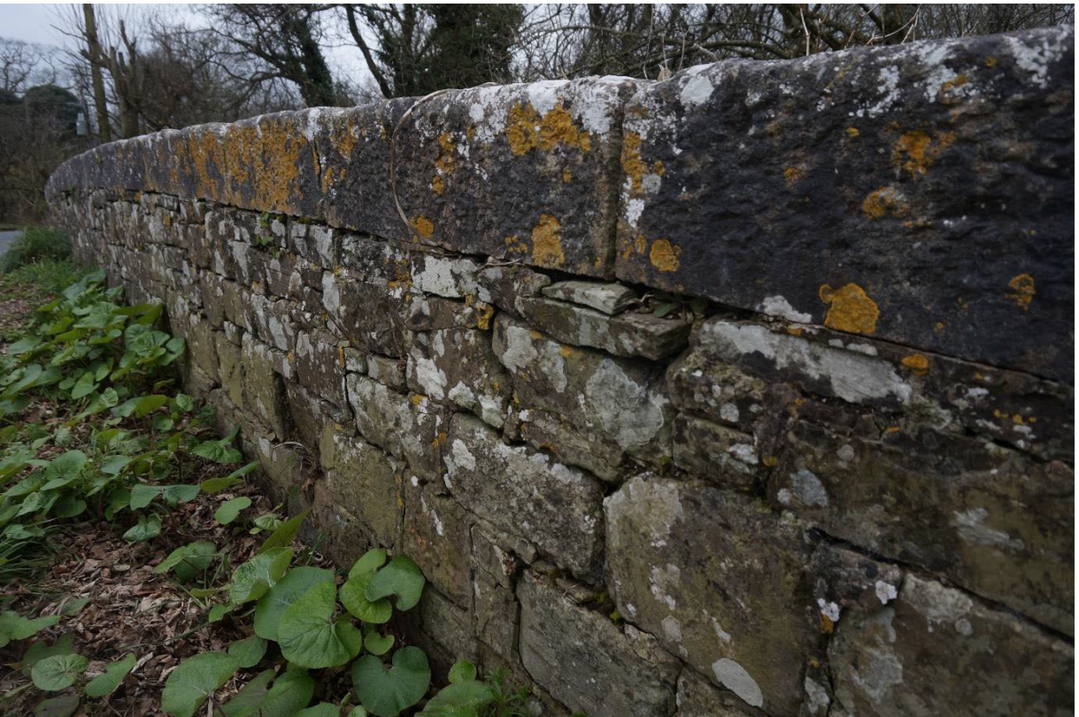
Loss of mortar pointing to mostly all parapet stonework and carbon soiling of stone surfaces
