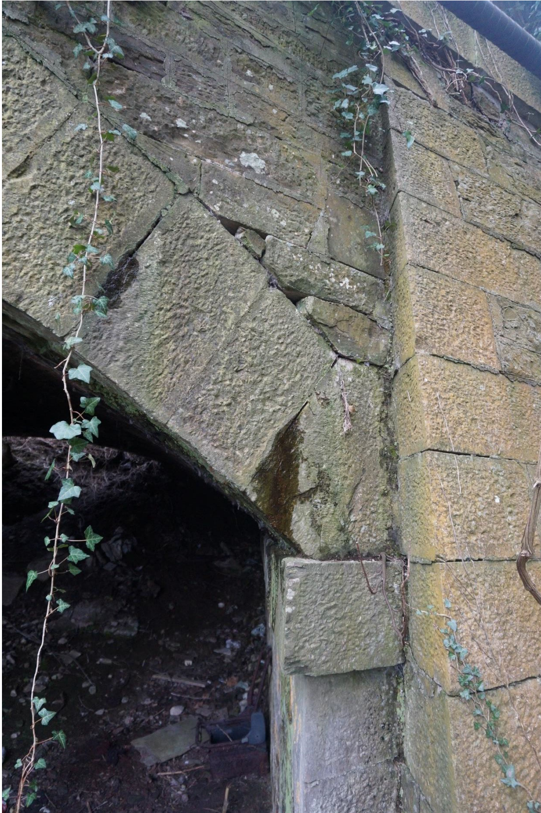
Detail of arch spring point: Considerable leaching of joints presumably caused by unsealed road surface and open stonework joints that have lost their mortar fill. Note the use of non-breathable cementitious mortars at the top of the photograph where the mortar is inappropriately brought over the stone face. Much of the ashlar stonework has lost its mortar fill.
