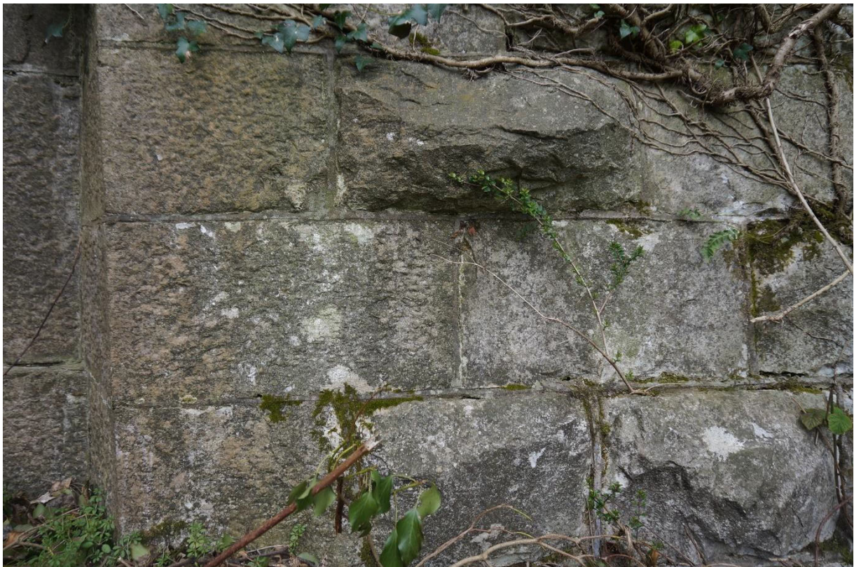
Detail of rusticated spandril stones. Note hard cement based pointing
