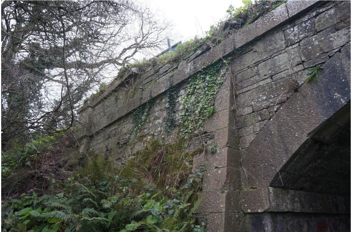
Detail of abutment and wing wall with severe loss of mortar pointing to stone joints
