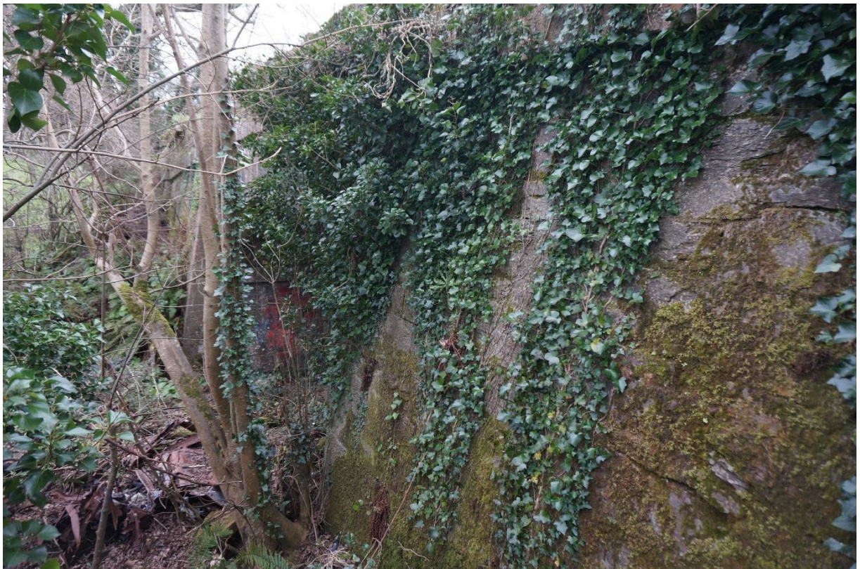
Extensive ivy overburden and tree growth on wing walls
