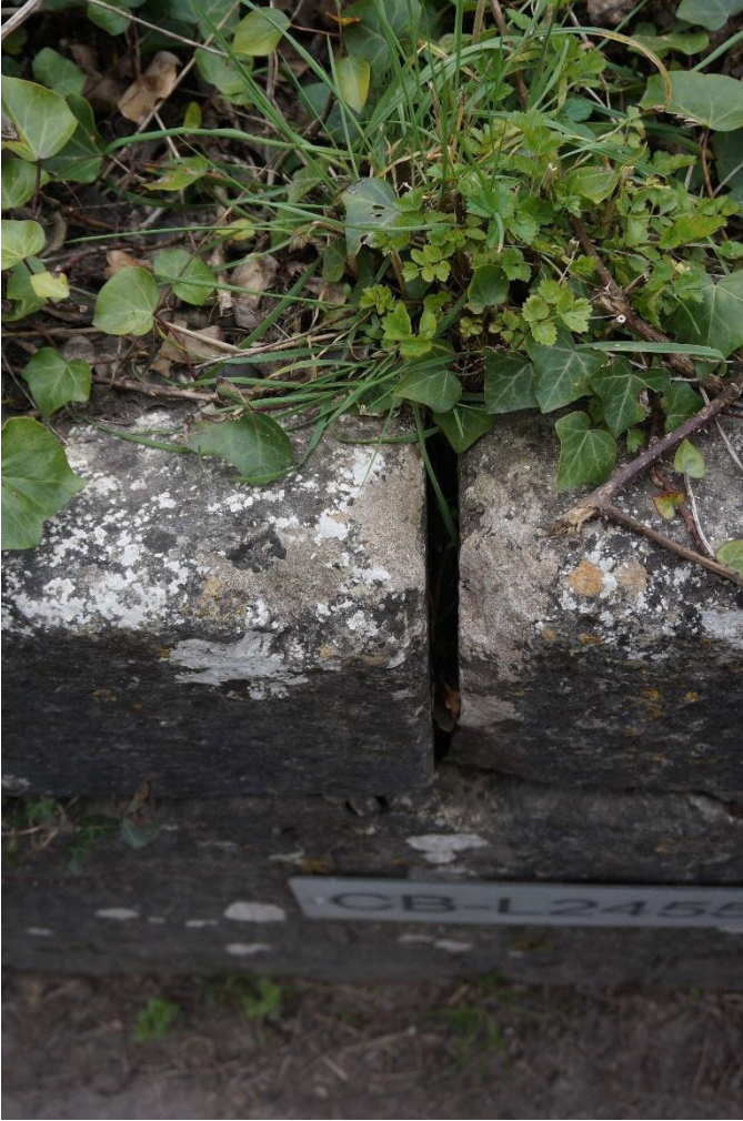
movement in parapet stones
