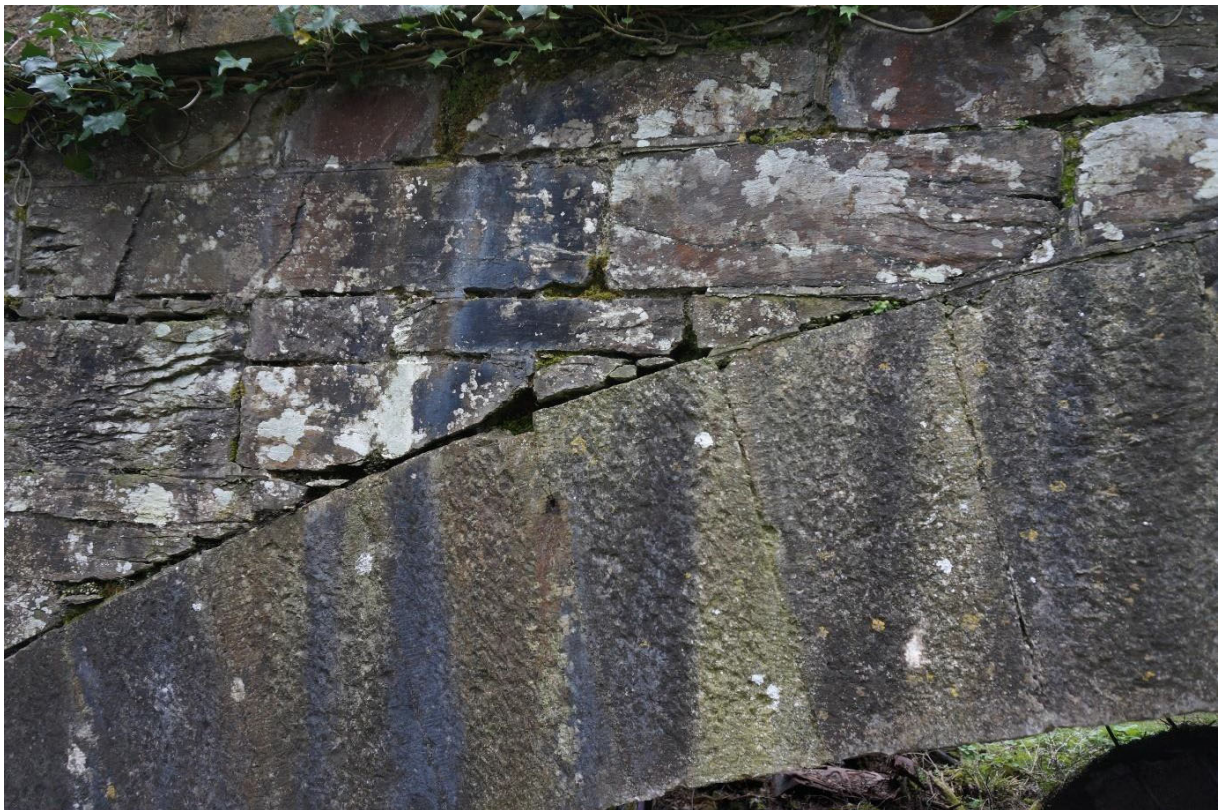
Loss of smaller stone pinnings and mortar pointing to spandrels above archline
