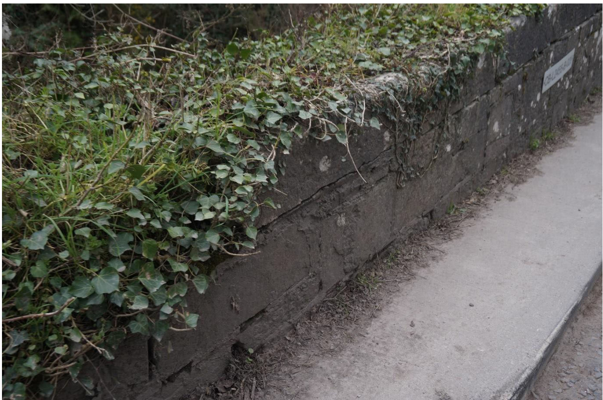
Considerable ivy overburden to bridge parapets
