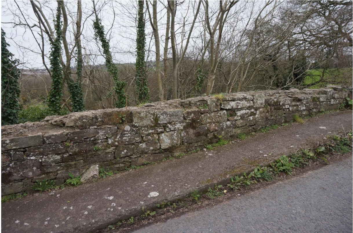
West Elevation of bridge parapet with coping and top rubble stone missing
