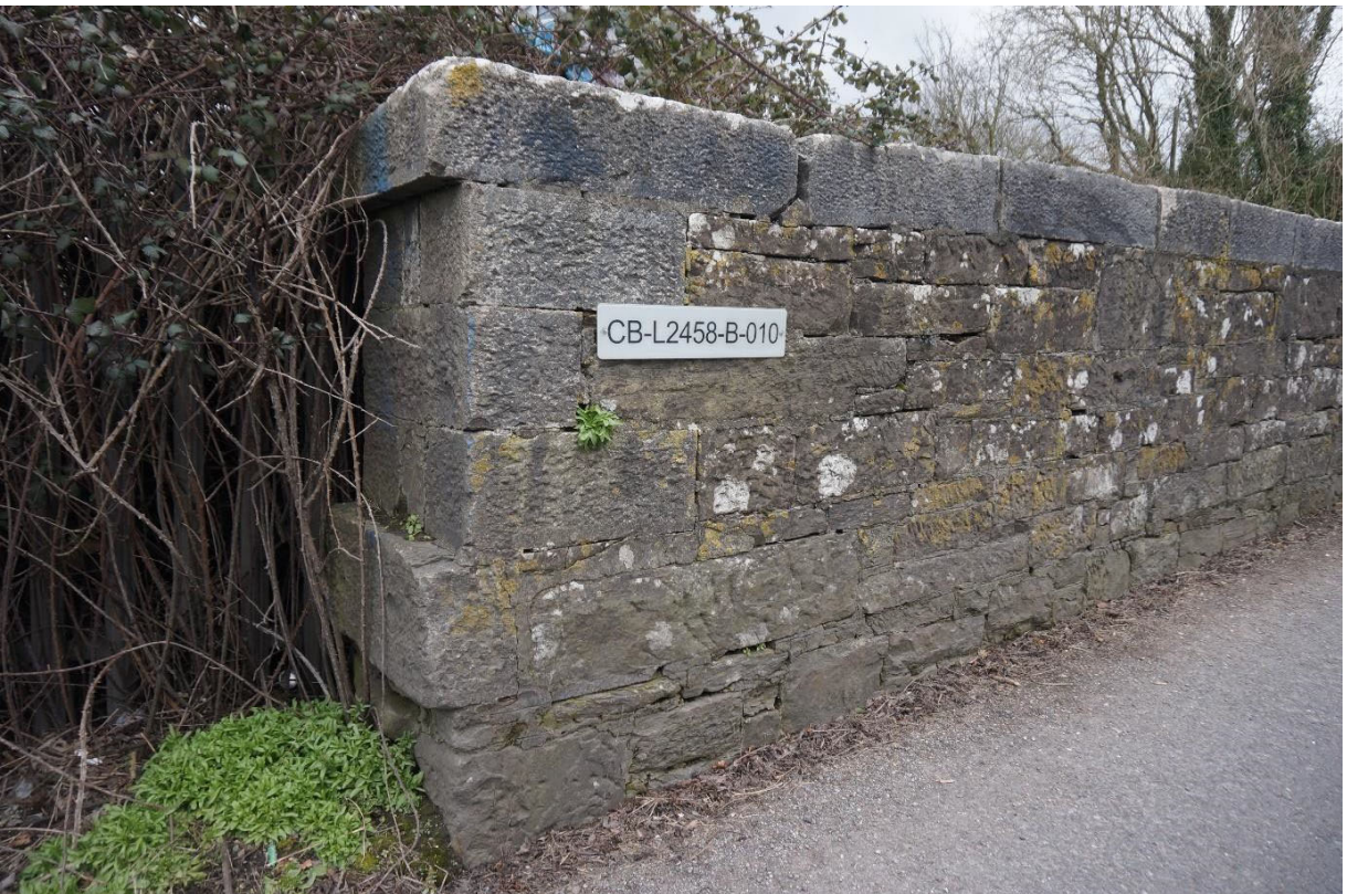
Loss of mortar pointing to ashlar stone capping and general parapet walling is evident
