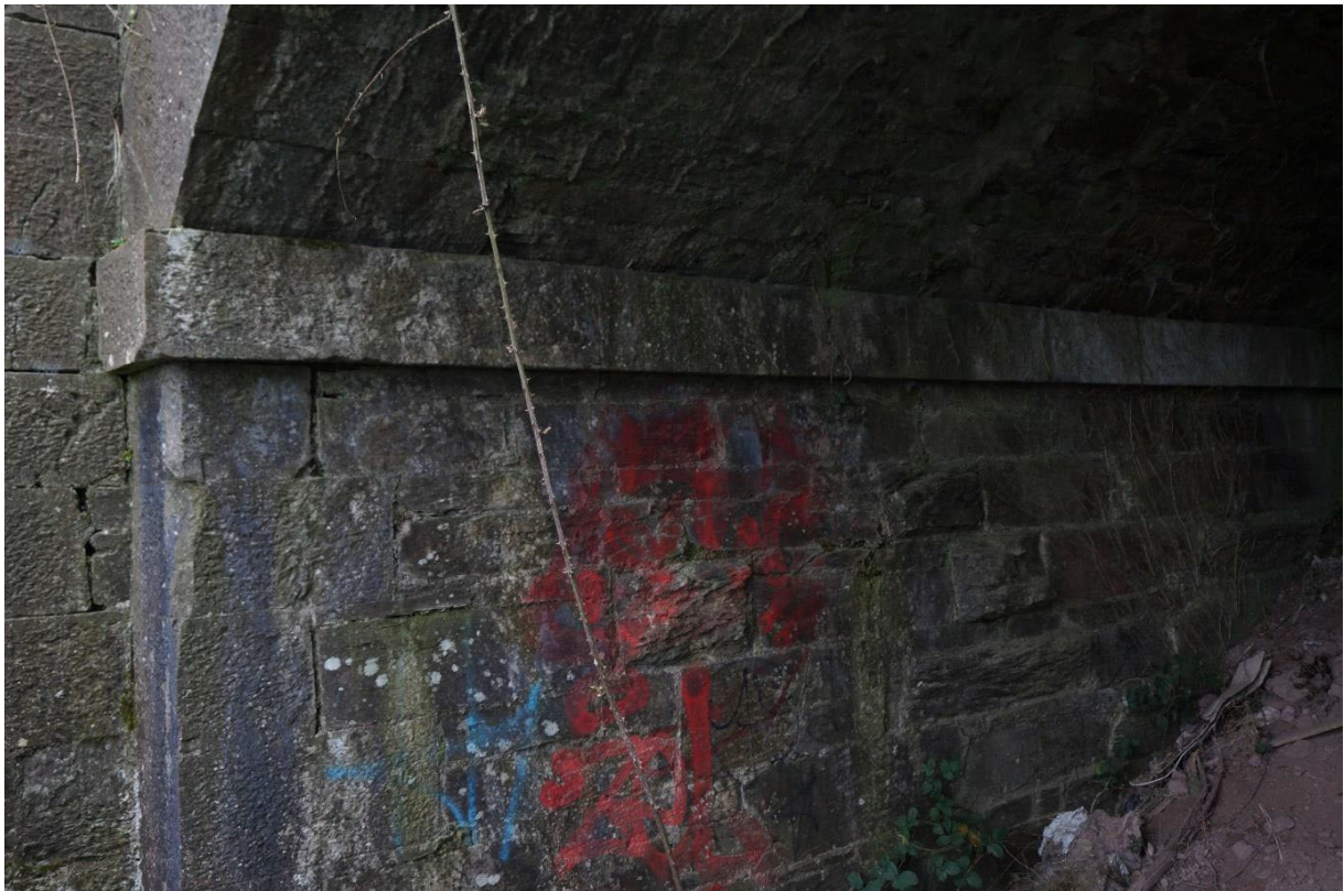
Stonework mortar joints are generally intact to the piers and vault barrel
