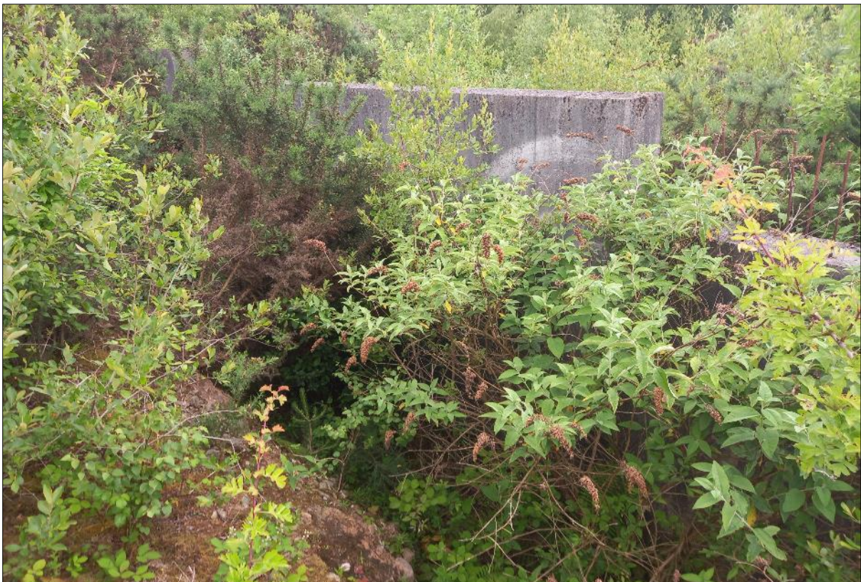
Plate 4: View of the concrete wall which extends across the central portion of the site in a roughly north to south direction
