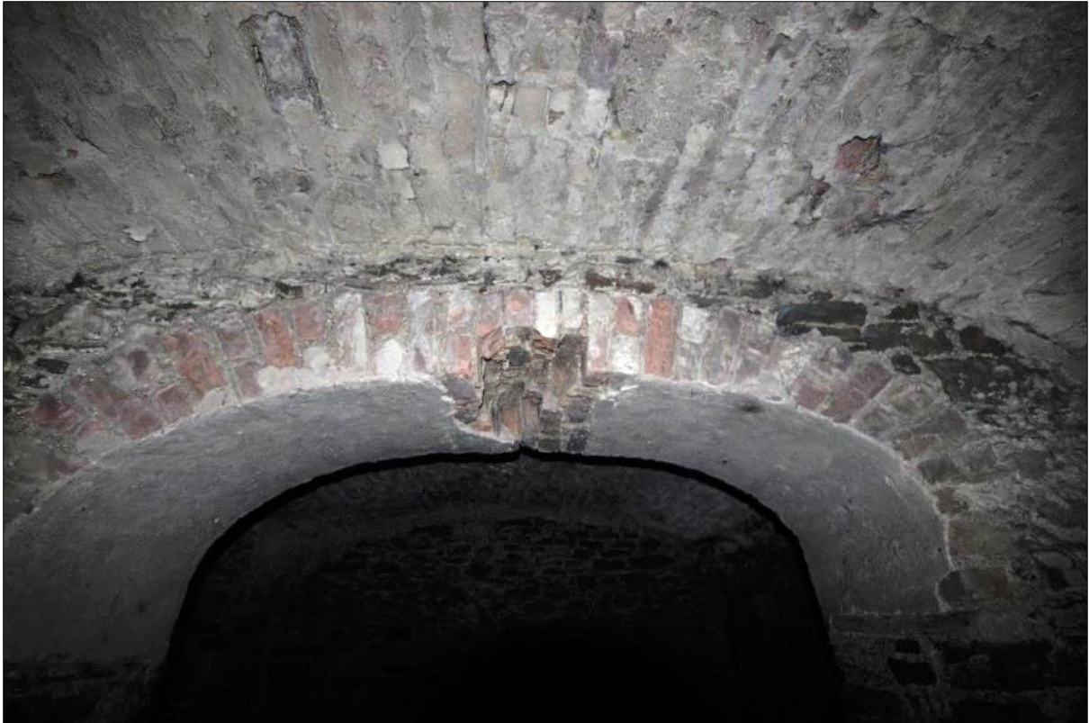
Plate 13: Missing bricks in arch on lower ground floor level LGF01
