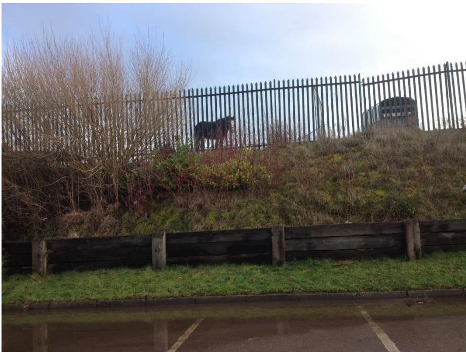
Fig 8 – Northside For Business Campus Eastern boundary after theft of panelling
