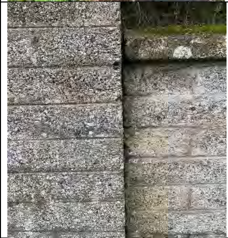
7. Separated joint between wall and pier
