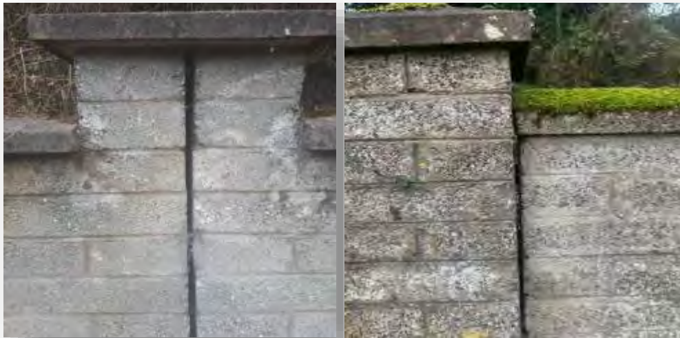
Figure 10 & 11: Separated joints (Refer to Appendix A&B for locations)
