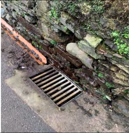
72. Loss of mortar, loose stones & water running through the bottom of the wall
