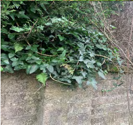
30. Top of pier is overgrown by vegetation & stain present on the face of the wall
