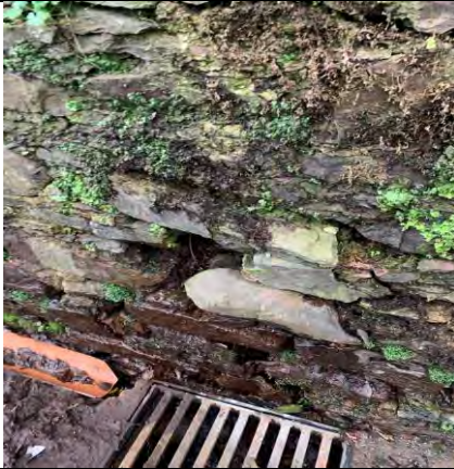
73. Loss of mortar and loss of stones & water running through the bottom of the wall
