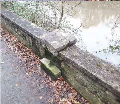
123. Loss of mortar&masonry to pier
