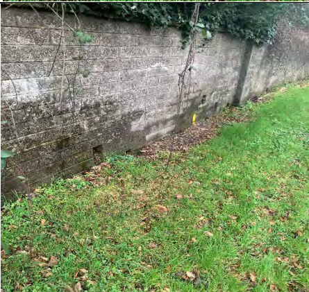
29. Water dripping through the bottom of the wall
