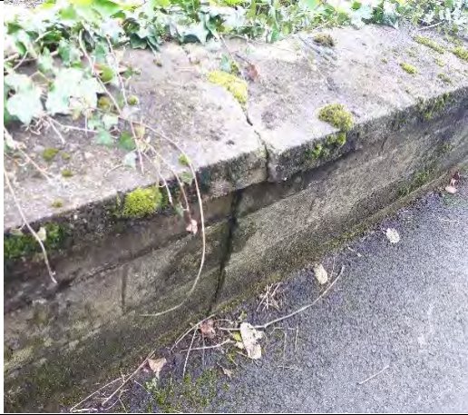
132. Crack&Deterioration of wall
