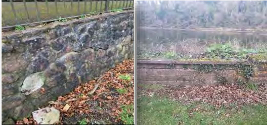
Figure 8 & 9: Horizontal cracks (Refer to Appendix A&B for locations)
