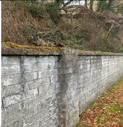
49. Top 2 courses of blockwork of pier collapsed
