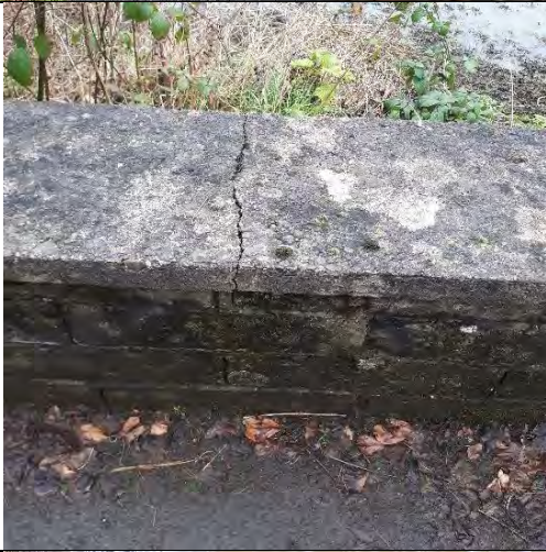
125. Vertical crack through wall
