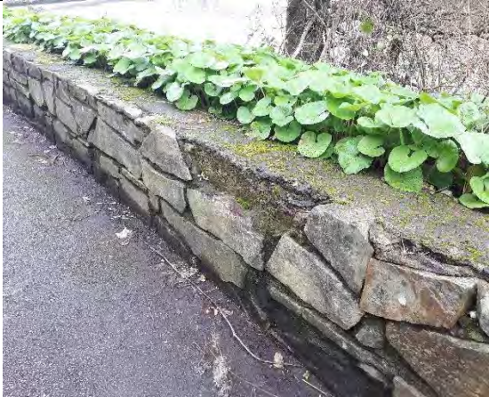
148. Loss of masonry&mortar
