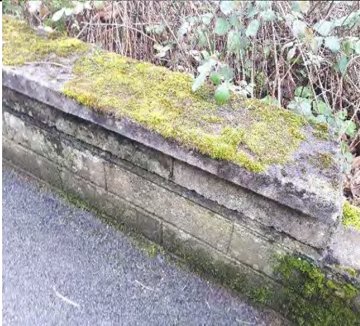
120. Crack through wall
