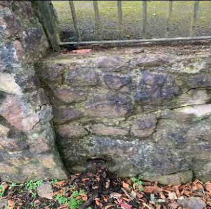
66. Horizontal crack through wall at entrance junction to the Cork's Vienna Hotel
