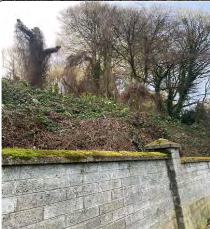
52. Gap between coping and wall
