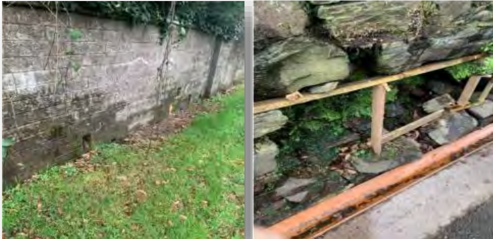
Figure 16 & 17: Loss of masonry & Collapsed wall (Refer to Appendix A&B for locations)
