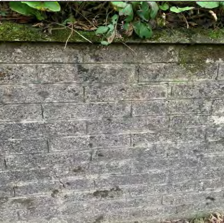
36. Vertical crack through wall
