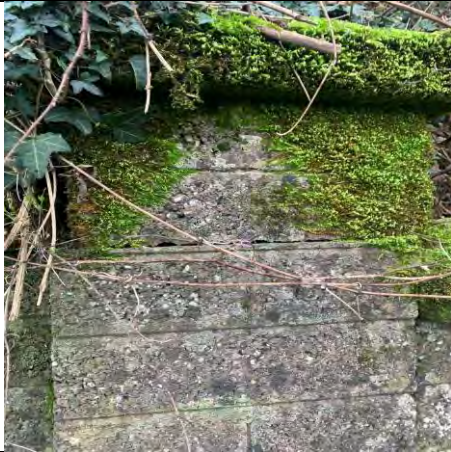
33. Top 2 course of blockwork of pier separated and moved & rotated
