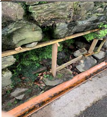
71. Evidence of loss of stones & mortar
