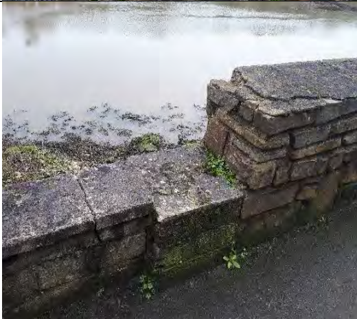
117. Loss of masonry
