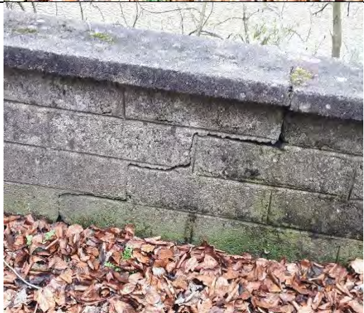
141. Vertical crack through wall
