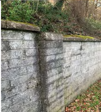
50. Top 2 courses of blockwork of pier collapsed
