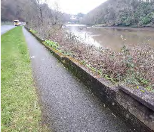
119. Collapsed wall section
