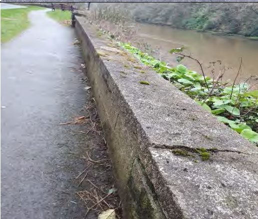
134. Crack&Deterioration of wall
