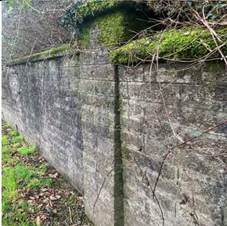
34. Wall beside pier tilting outwards
