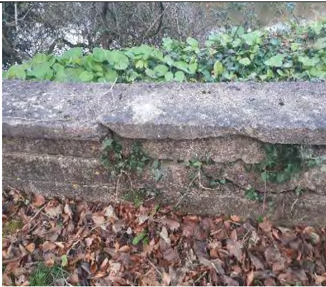
96. Crack through wall & coping Spalling of concrete on coping
