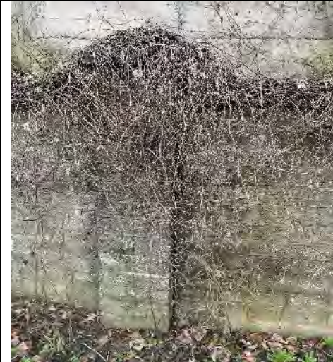
13. Pier overgrown by vegetation
