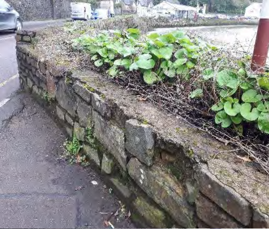
150. Loss of masonry&mortar
