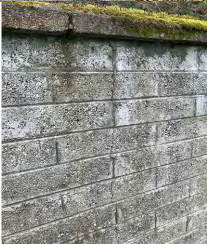
51. Vertical crack through wall
