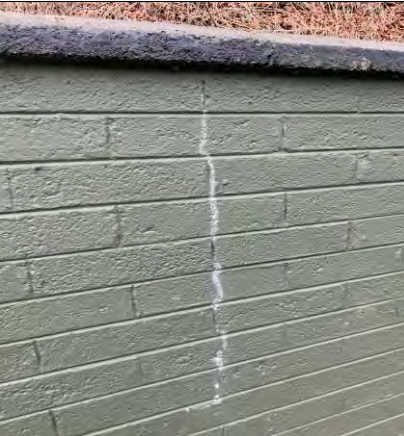
62. Vertical crack through wall
