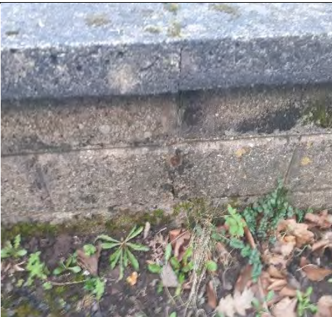
97. Vertical crack through wall & coping
