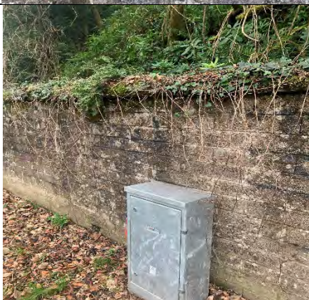
23. Gap between coping and top of wall & vegetation growth to wall
