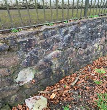
65. Horizontal crack through wall at entrance junction to the Cork's Vienna Hotel
