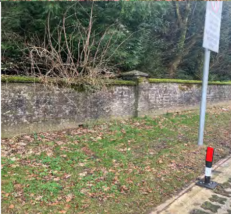
25. General view to the wall & vegetation growth to the coping & sign of stain on wall
