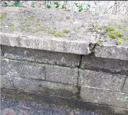
131. Vertical crack through wall
