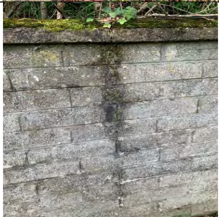
47. Water seeping through wall
