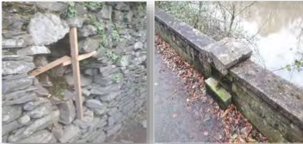
Figure 14 & 15: Loss of masonry (Refer to Appendix A&B for locations)
