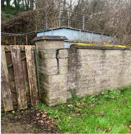
16. Serious deterioration of pier
