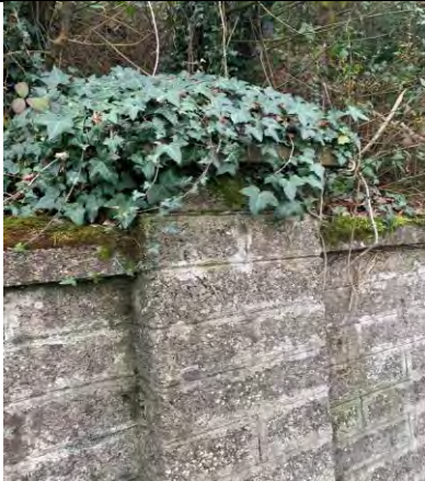
37. Division of top part of pier under first course of blockwork & top of pier covered with vegetation
