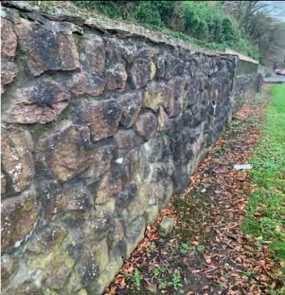
64. Horizontal crack through wall at entrance junction to the Cork's Vienna Hotel
