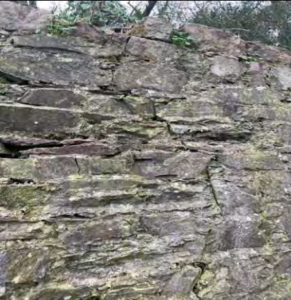
74. Vertical crack through wall
