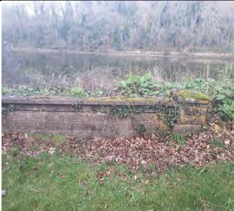
95. Crack through & deterioration of pier and adjacent wall
