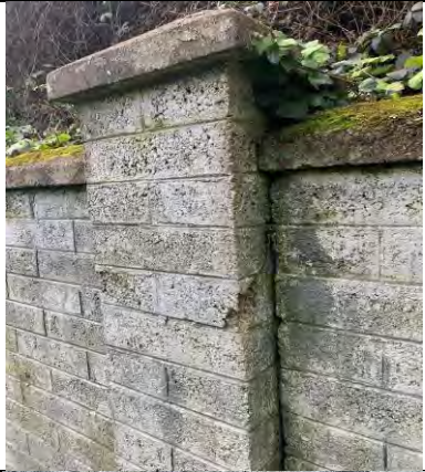
59. Separated vertical joint between the pier and the wall
