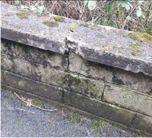
121. Crack through wall
