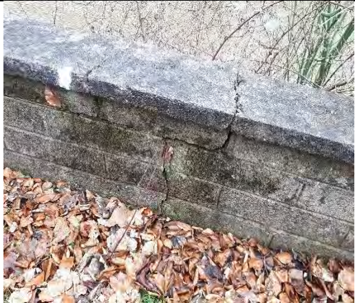
140. Vertical crack through wall
