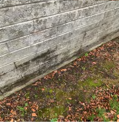
61. Evidence of stain on bottom face of the wall
