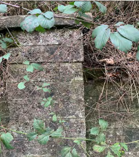
31. Top of pier separated under the top course of block and moved
