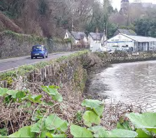
151. Evidence of tree growth to rear of wall
