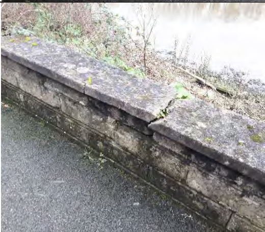
118. Crack through wall & tilting wall
