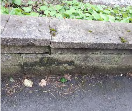
133. Crack&Deterioration of wall
