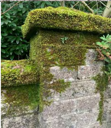
38. Top part of pier separated under the first blockwork and moved & pier covered by vegetation
