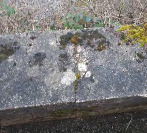
98. Crack & minor vegetation on coping
