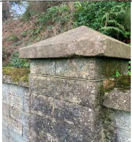
48. Top block course of pier separated and moved
