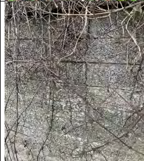
14. Vertical crack through wall
