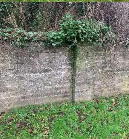
19. Top of pier overgrown by vegetation & separated joint between wall and pier
