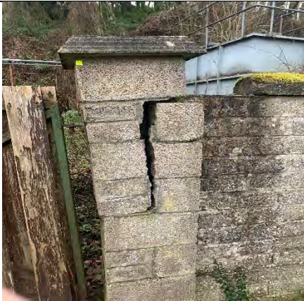
17. Cracked top part of pier tilting out & missing coping
