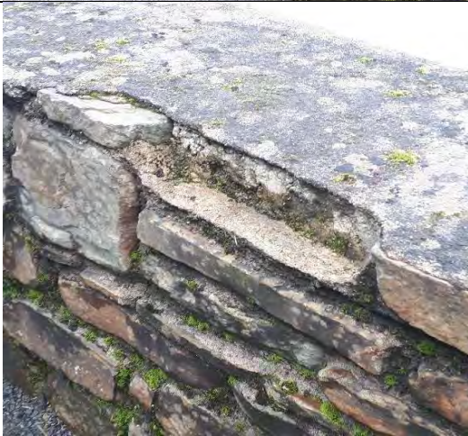
116. Loss of masonry
