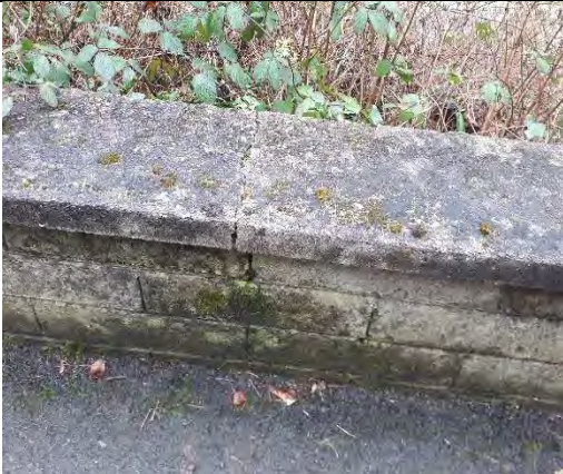
128. Vertical crack through wall
