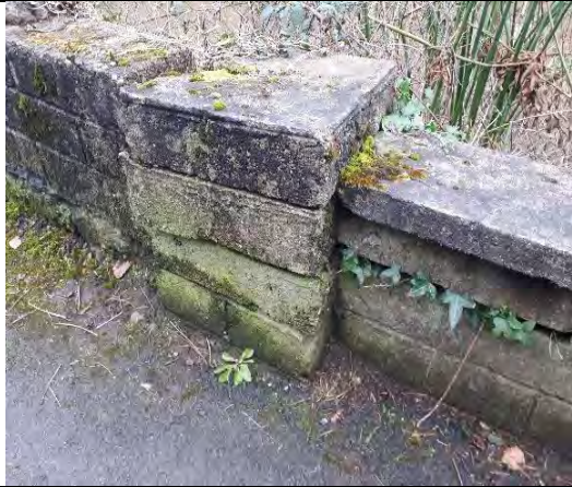
135. Crack&Deterioration of pier & missing coping
