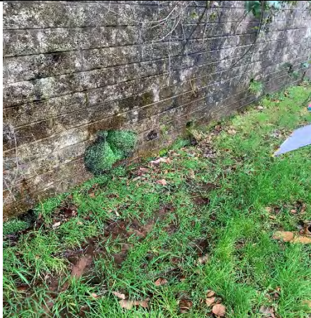
28. Water dripping through the bottom of the wall. The ground in front of the wall is soaked
