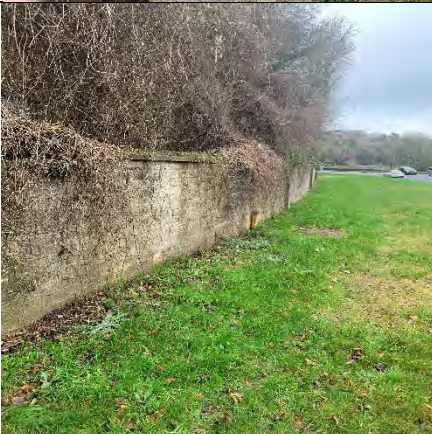
18. Wall overgrown by vegetation
