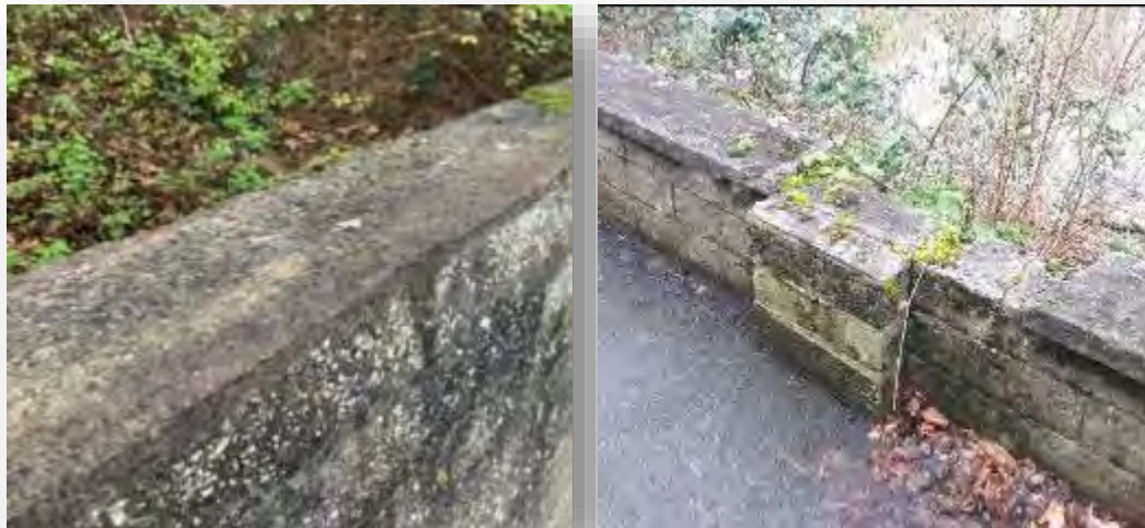
Figure 21 & 22: Collapsed structure (Refer to Appendix A&B for locations)
