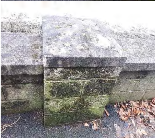
127. Horizontal crack on pier
