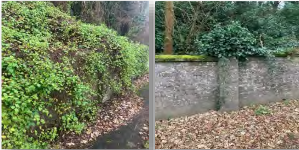
Figure 2 & 3: Wall overgrown by vegetation (Refer to Appendix A&B for locations)
