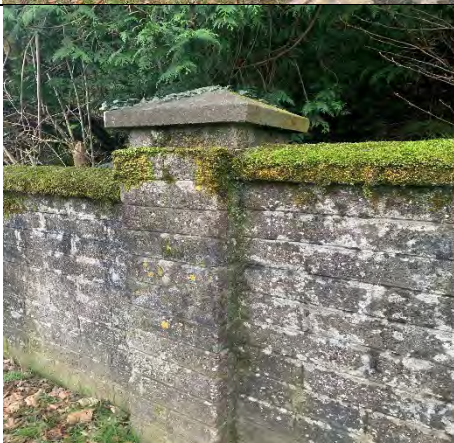
26. Structural division of top course of block of the pier separated and moved
