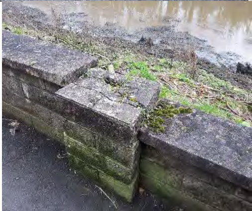
129. Top of pier collapsed & cracked
