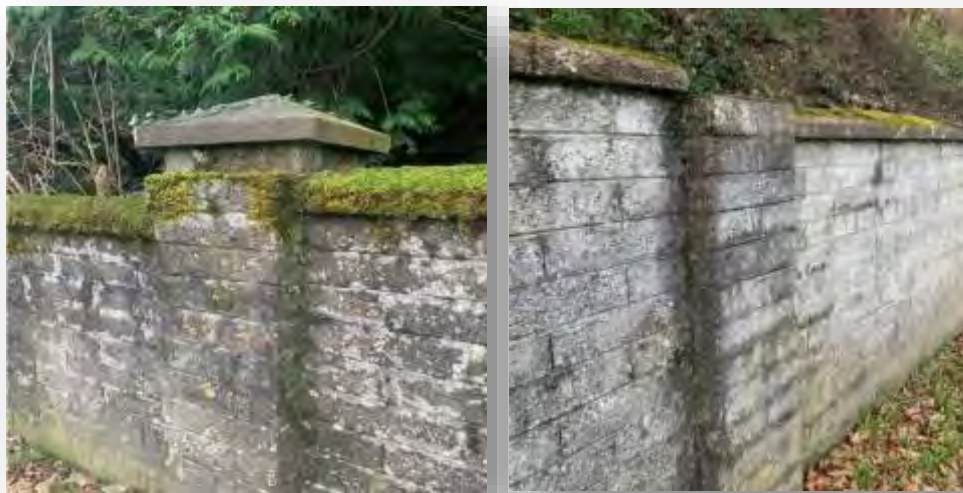
Figure 4 & 5: Damage to piers (Refer to Appendix A&B for locations)
