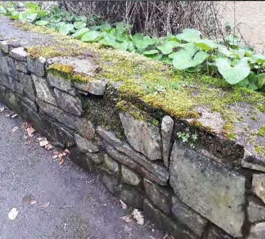
145. Loss of mortar&masonry
