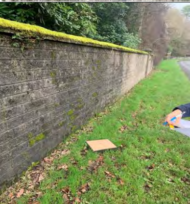
39. Stain present on the face of the wall
