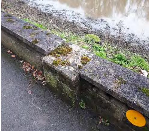
126. Loss of masonry & coping to pier
