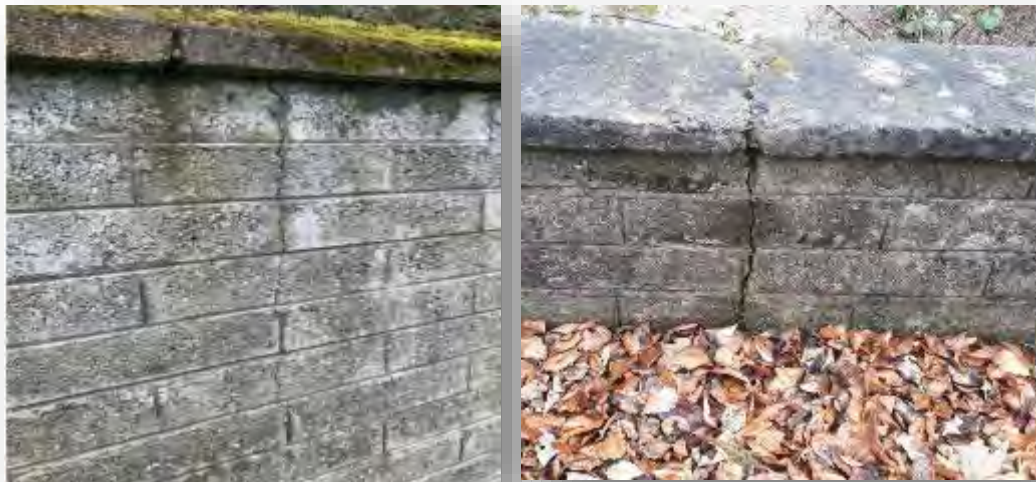
Figure 6 & 7: Vertical cracks (Refer to Appendix A&B for locations)
