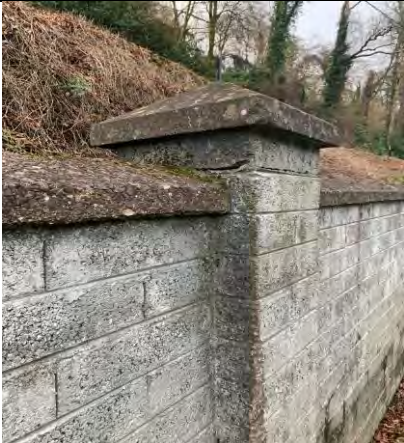
60. Horizontal crack at top of pier
