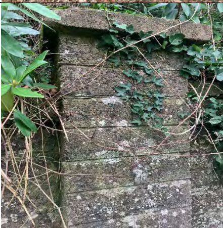
22. Horizontal crack through mortar at top of pier & vegetation growth
