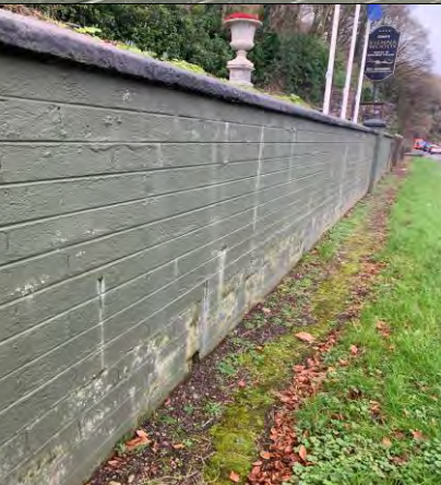
63. Water seeping through the bottom of the wall throughout
