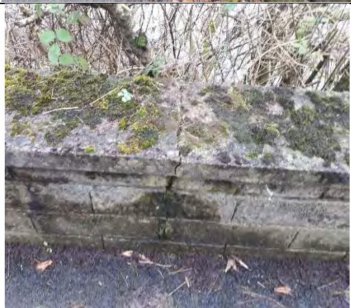
124. Vertical crack through wall
