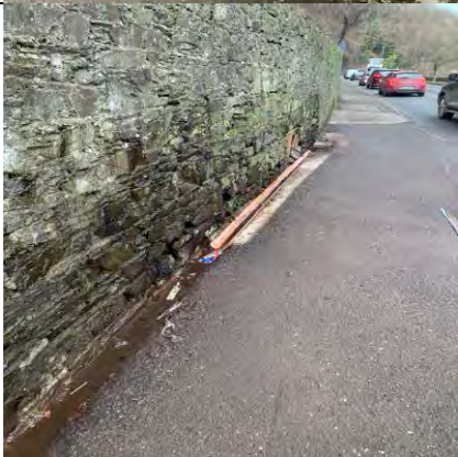
70. Water broke through wall & bottom of wall soaked
