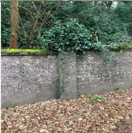
21. Top of pier overgrown by vegetation
