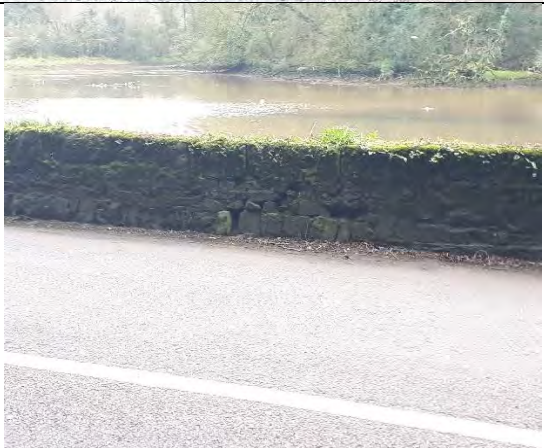
153. Loss of masonry&mortar
