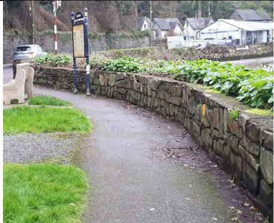
149. Loss of masonry&mortar
