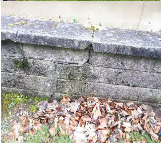
137. Vertical crack through wall
