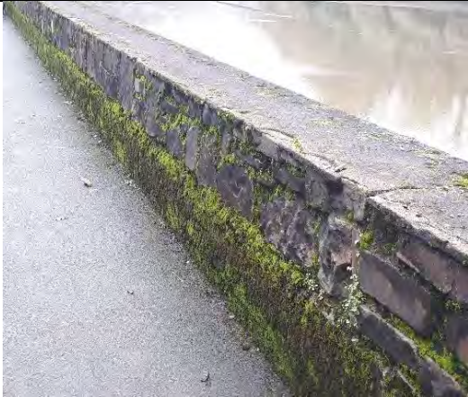
115. Vegetation growth to the bottom of wall
