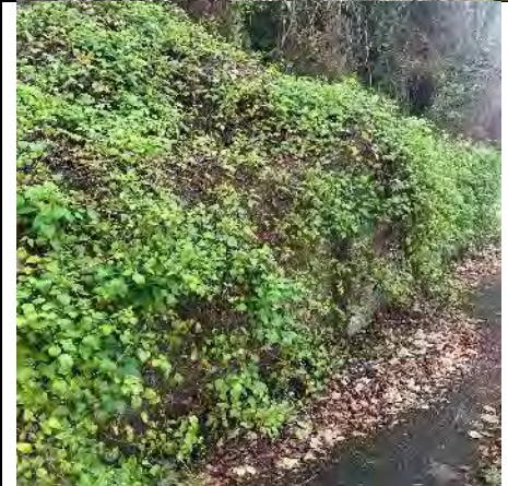
6. Wall heavily overgrown by vegetation
