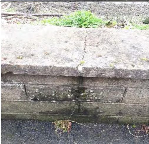
130. Vertical crack through wall
