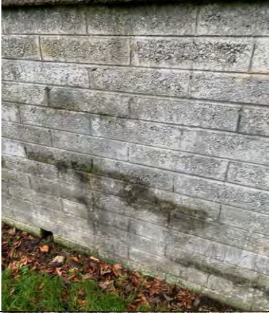
57. Evidence of weephole & Water seeping through wall
