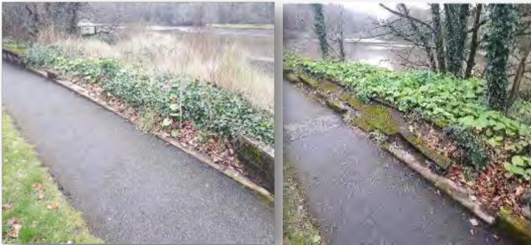
Figure 20 & 21: Collapsed structure (Refer to Appendix A&B for locations)
