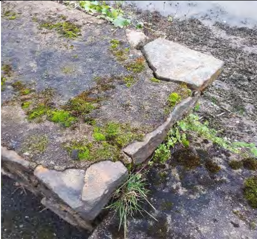
111. Loss of mortar & loose masonry at the edge of stone wall
