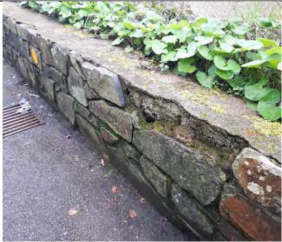
147. Loss of masonry&mortar
