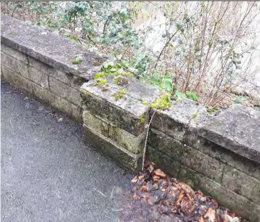
122. Top of pier collapsed
