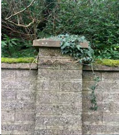
41. Horizontal crack through mortar at top of pier
