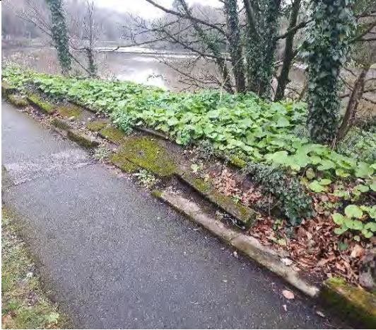
108. Collapsed section of wall
