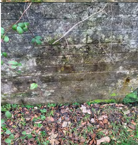
27. Water seeping through the wall
