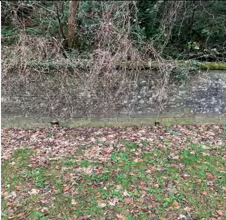
24. Blocked weepholes at bottom of wall & vegetation growth to wall
