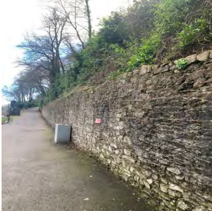
69. Entrance road to Cork's Vienna hotel & loss of mortar and loose stones evident
