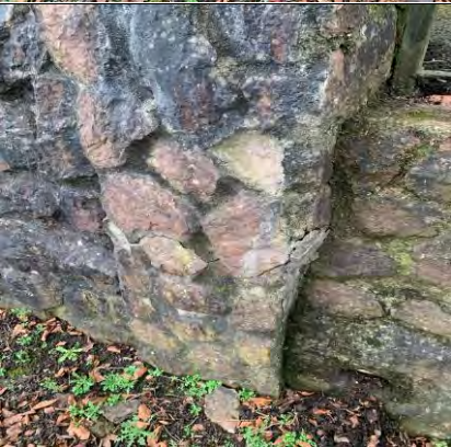
67. Horizontal crack through wall at entrance junction to the Cork's Vienna Hotel
