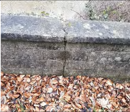
139. Vertical crack through wall
