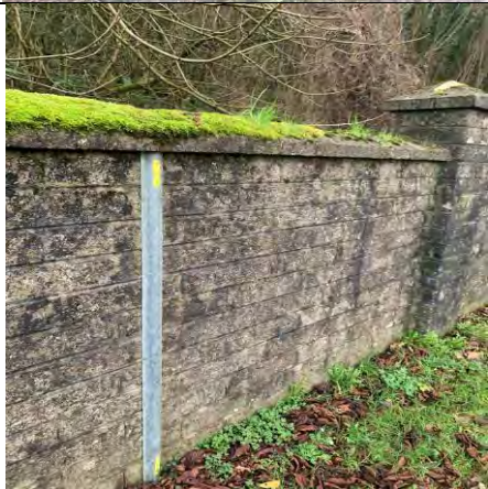
46. Electrical cable fixed to wall & evidence of stain present throughout
