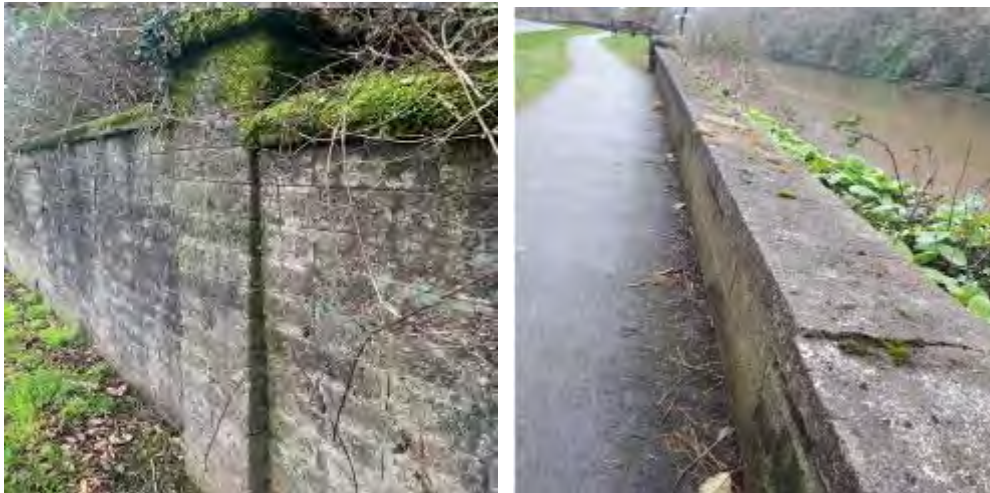
Figure 18 & 19: Wall leaning (Refer to Appendix A&B for locations)
