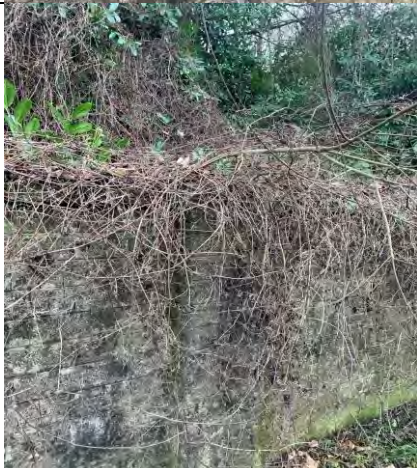
44. Top of pier collapsed & vegetation growth onto it & stain present on the face of the wall throughout
