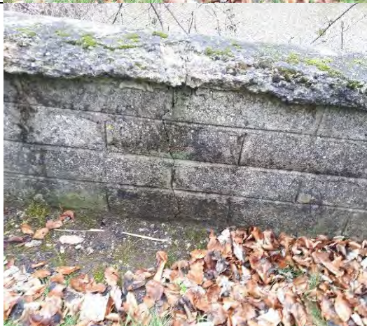
138. Vertical crack through wall & spalling of concrete on coping
