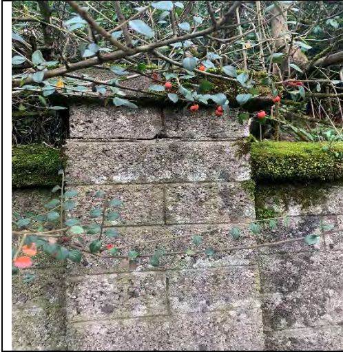
32. Top of pier separated under the top course of block and moved
