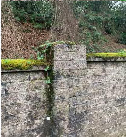
43. Missing coping on pier & stain present on the face of wall throughout
