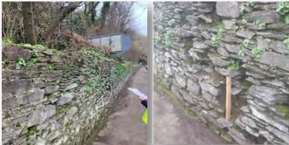
Figure 12 & 13: Loss of mortar (Refer to Appendix A&B for locations)
