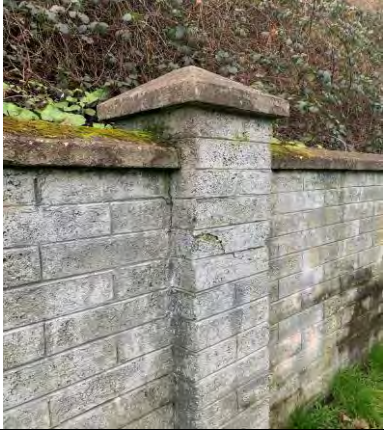
58. Horizontal crack through pier & evidence of stain on face of wall
