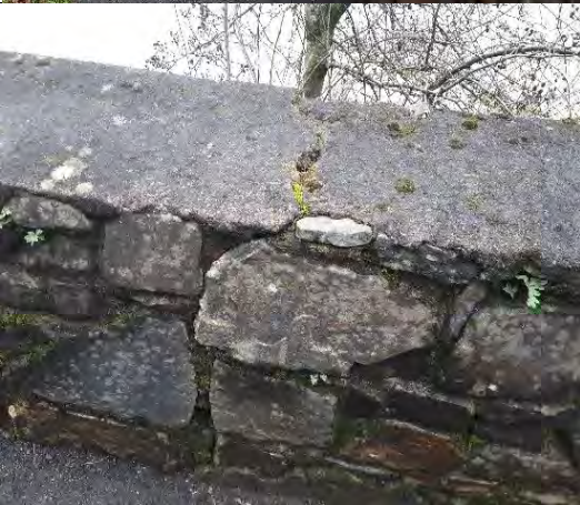
113. Crack on render
