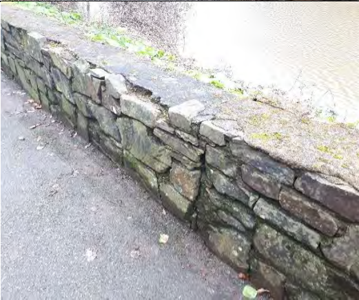
144. Loss of mortar&masonry
