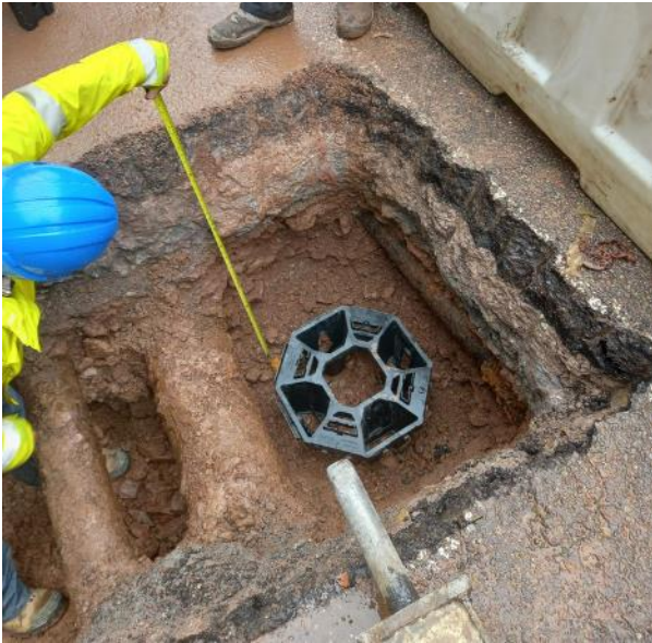
Figure 6.2 Underground services on MacCurtain Street limited the area available for tree planting
