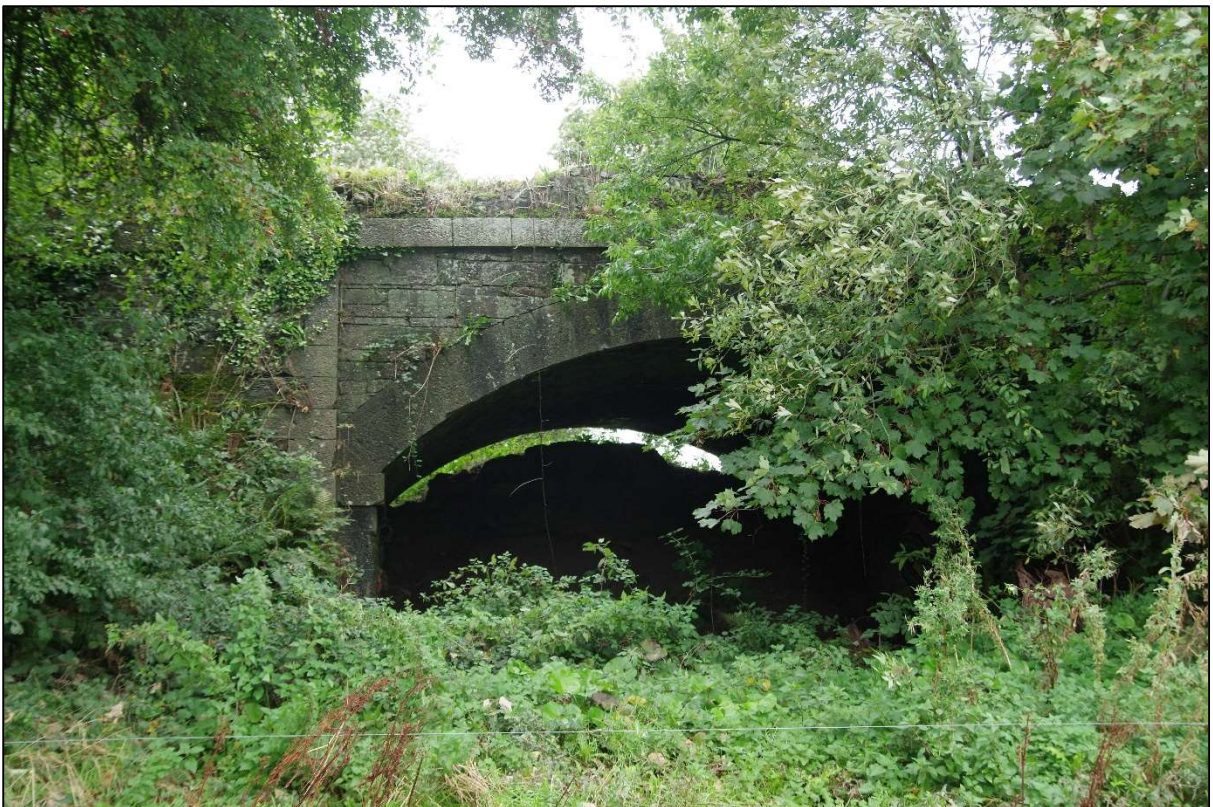
Plate 2: View of Spur Hill railway bridge from east with overgrowth and soil dump visible
